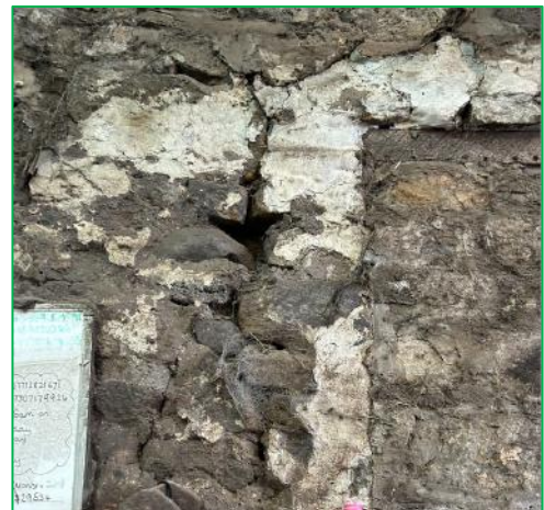
One of a small number of holes in the internal wall in the eastern half
