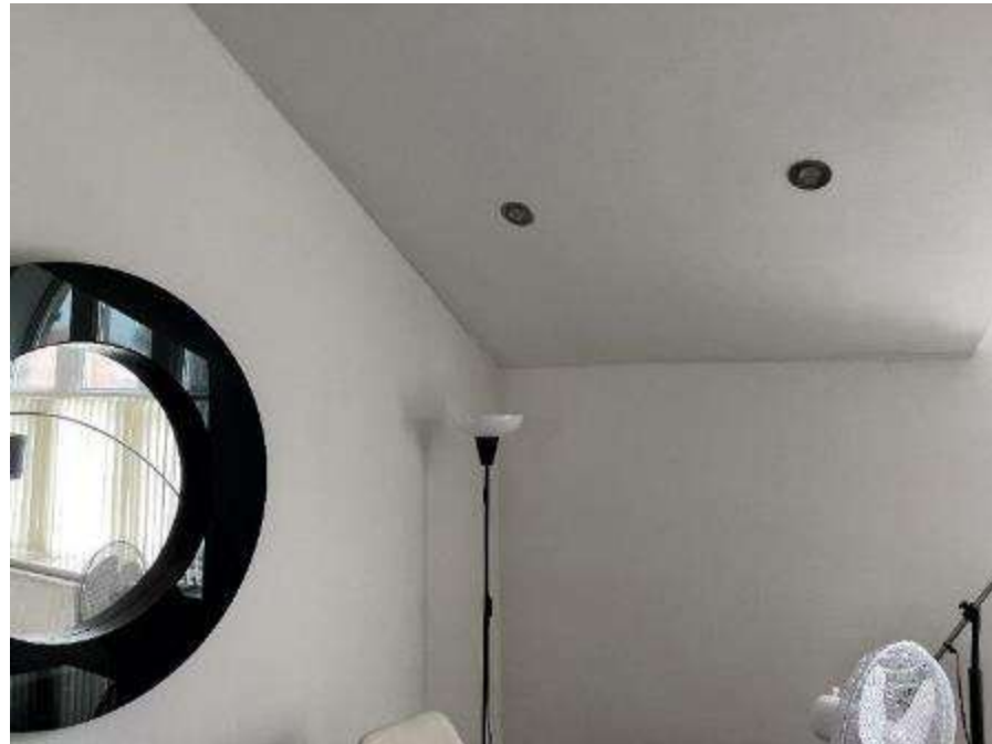
Figure 19 – Minor Cracking at Junction Between Wall and Ceiling (Non-Structural Shrinkage Cracking)
