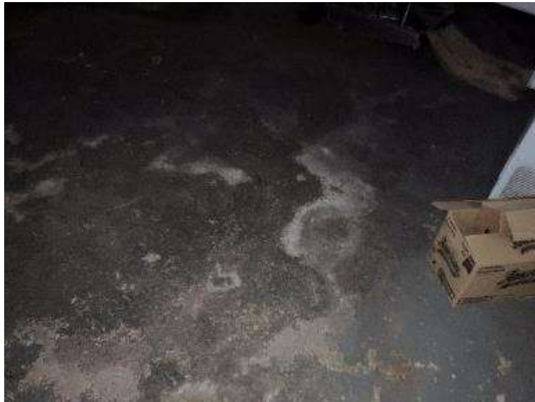
Figure 8 – Possible Damp Staining to Basement Floor
