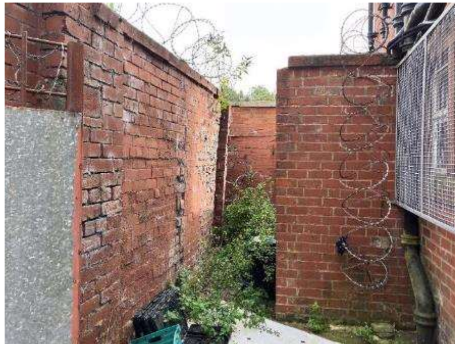
Figure 22 – View on Leaning Section of Yard Wall
