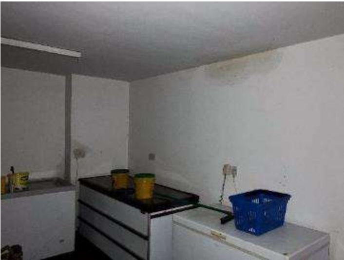
Figure 6 – Possible Damp Staining to Basement Wall
