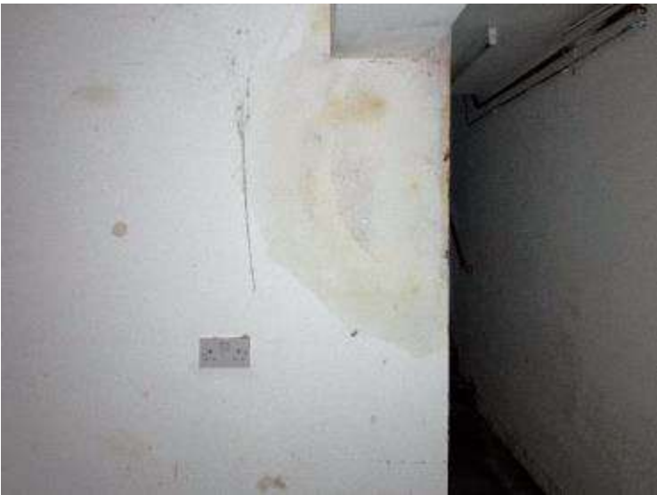
Figure 7 – Possible Damp Staining to Basement Wall
