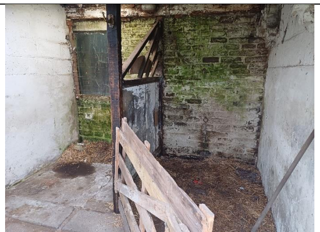
Photograph 12: Stains on flagged floor not of hydrocarbon origin.
