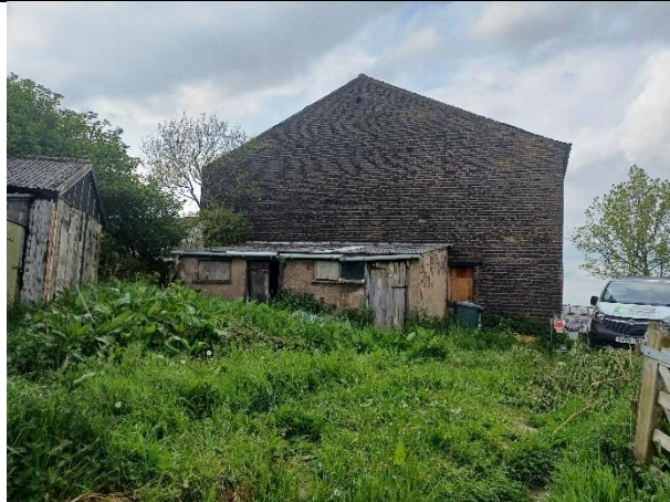
Photograph 3: Outbuildings in poor repair and vegetation with no sign of stress.
