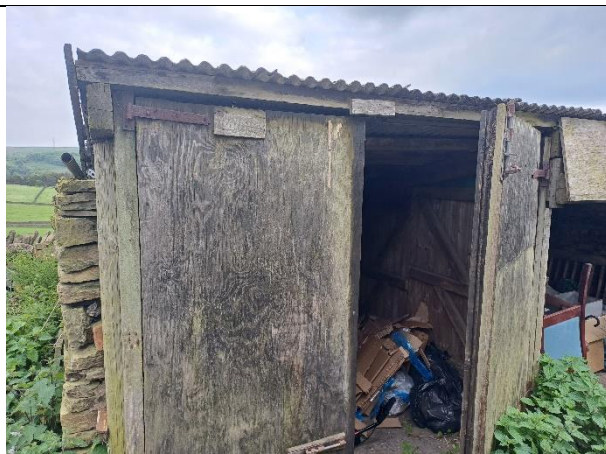
Photograph 5: The outbuildings appear to have been used to store household waste in the east of the site.
