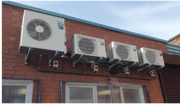
Figure 4 Installed condenser units
