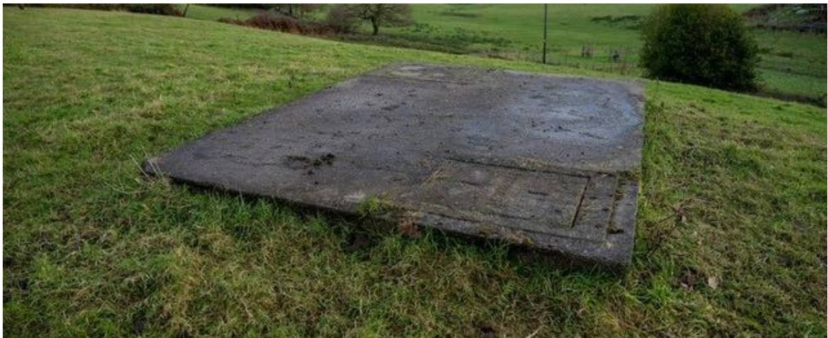
Fig. 12. Field Septic Tank
