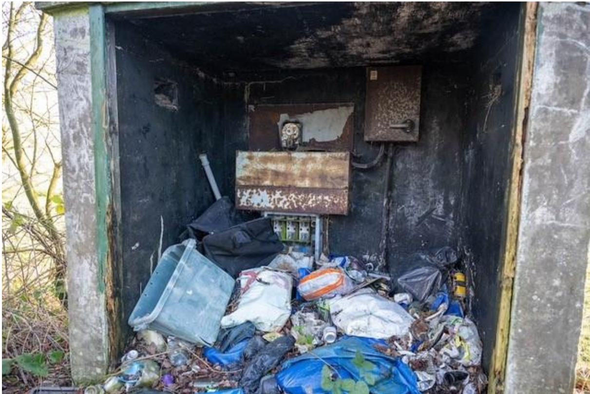
Figs. 1 & 2. Electricity Supply Cabinet with switchgear.
