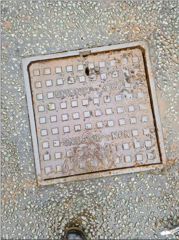
MH2 Cover Condition View
