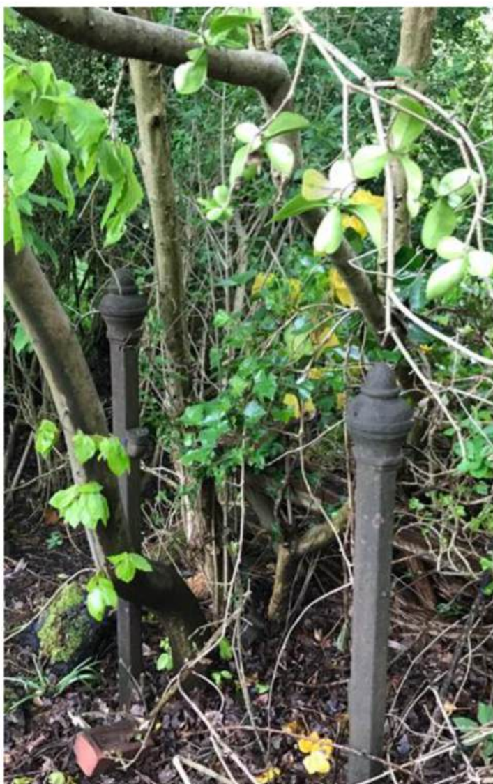
Cast iron posts
