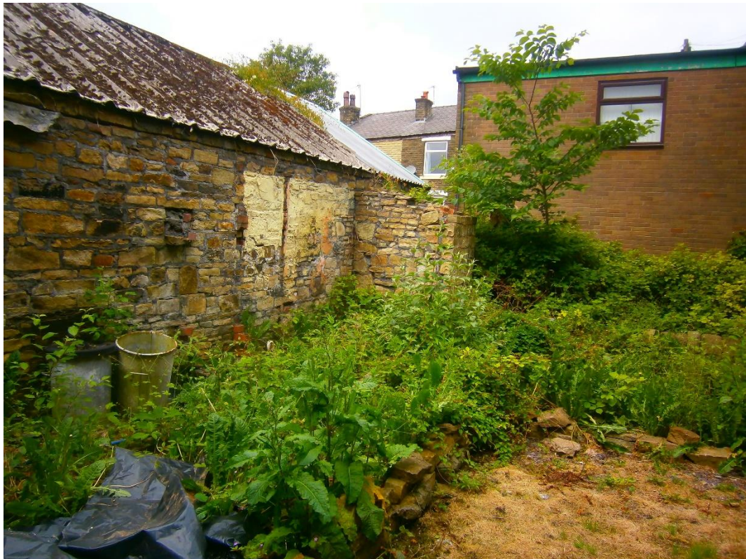
Rear elevation of garage partly demolished due to condition
