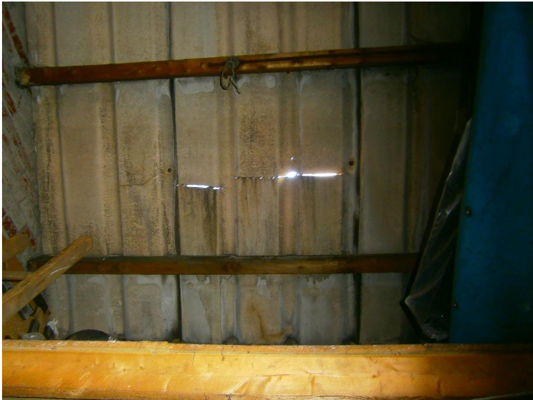
Damaged asbestos roof
