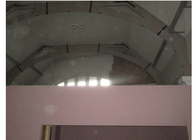
Photo 5. North wall below RF03.
