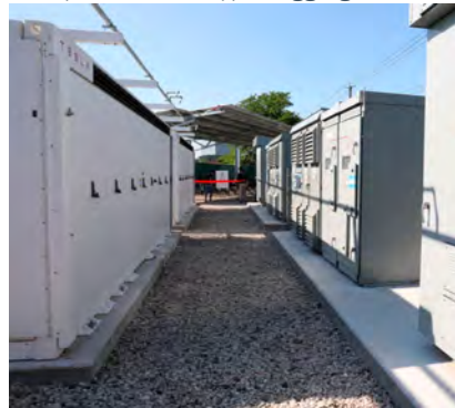
Battery storage units in greys
