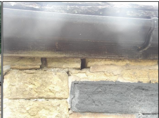
Figure 7: Voids behind the fascia boards.
