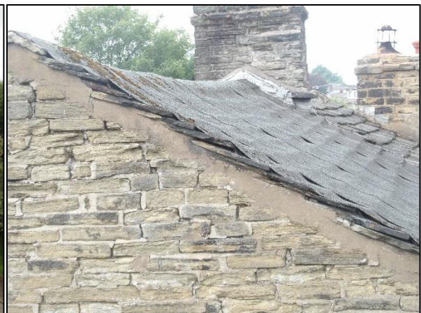
Figure 9: Voids along the verge of the building.
