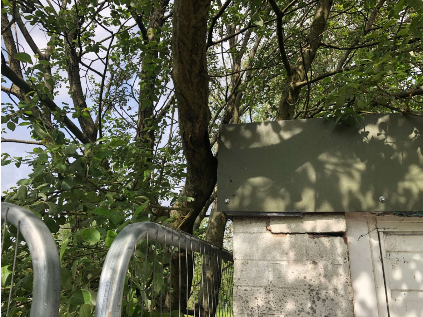
Branch on T4 rubbing on garage.
