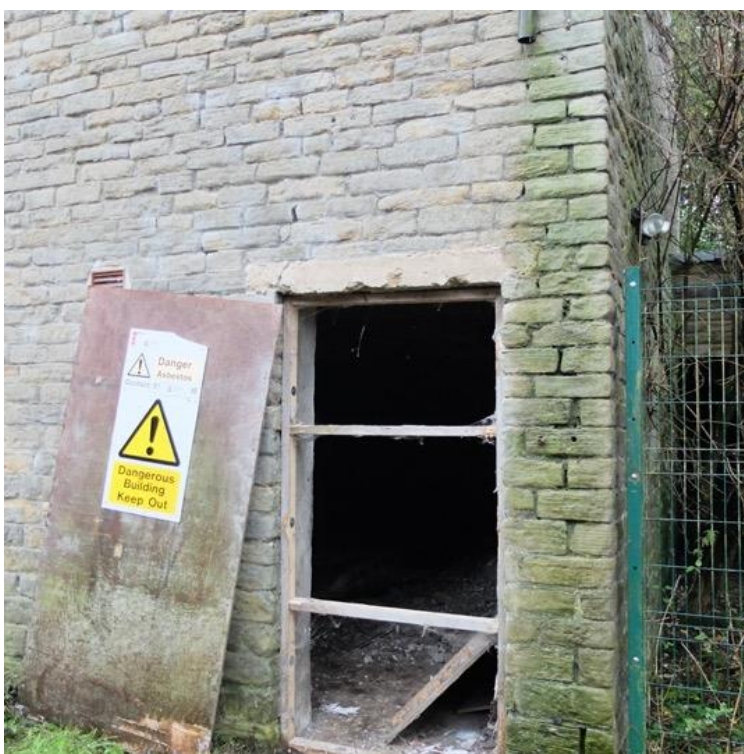
Photo. Damaged stone lintel above door
