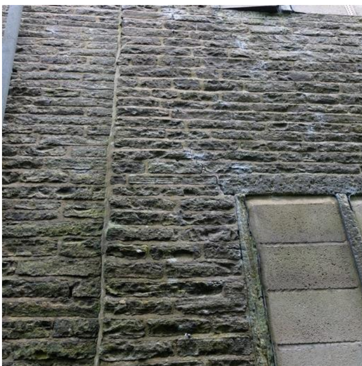
Photo. Diagonal crack above ground floor window to extension
