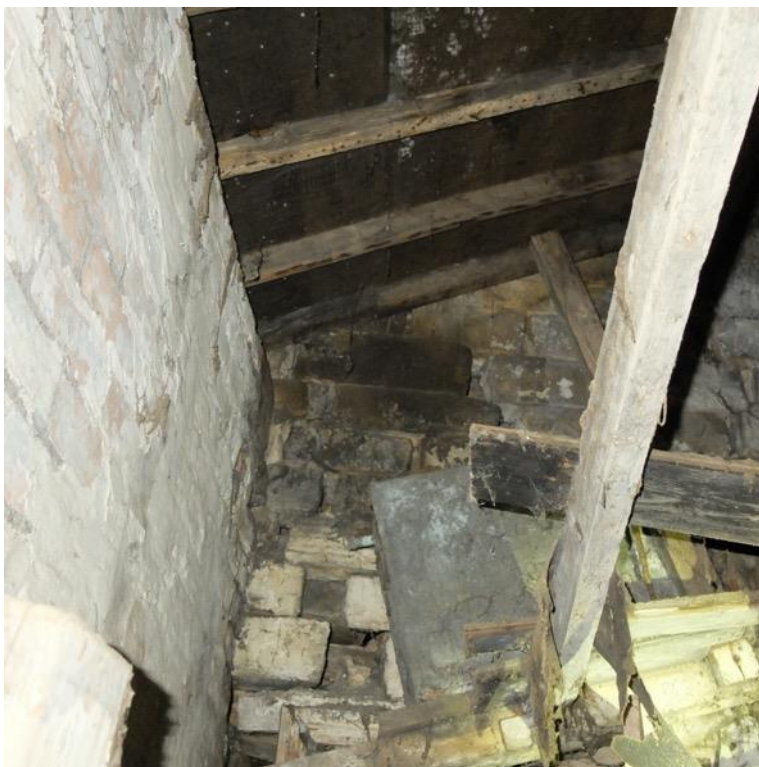
Photo. Movement above doorway which extends up to roof (photo above) outward movement of brick walls
