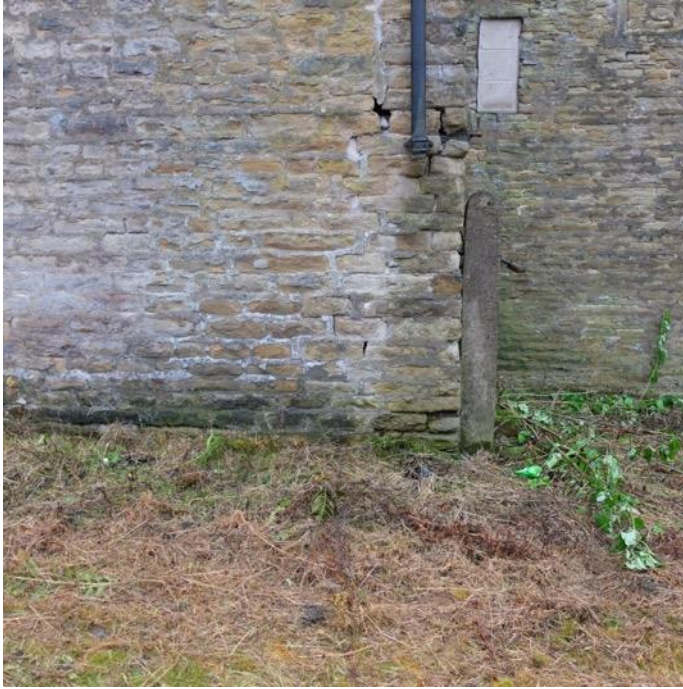
Photo. Eroded stonework to corner in location of downspout, foundation investigation required
