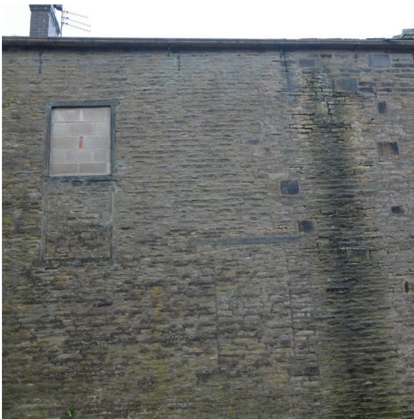
Photo. Infilled windows to rear elevation.
