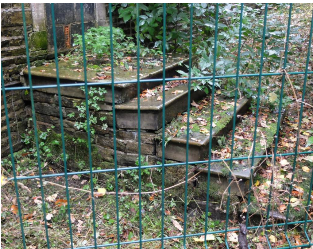
Photo. Stone steps to front door require repair.
