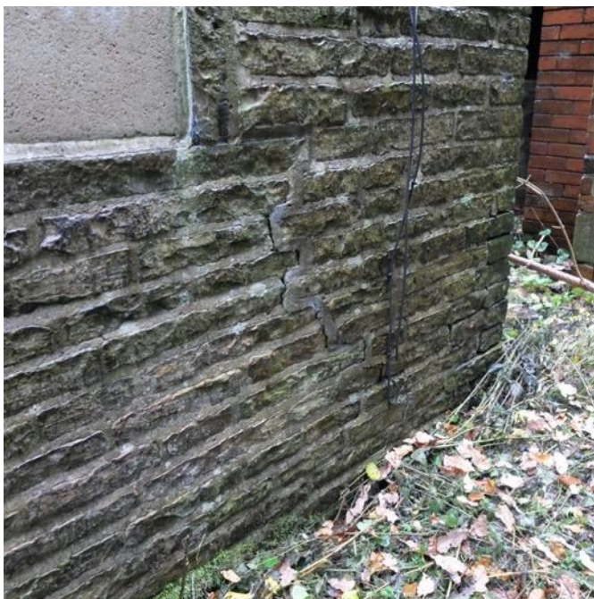
Photo. Diagonal cracking towards front right corner
