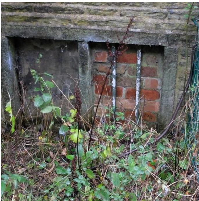
Photo. Bars to basement window concern regarding corrosion
