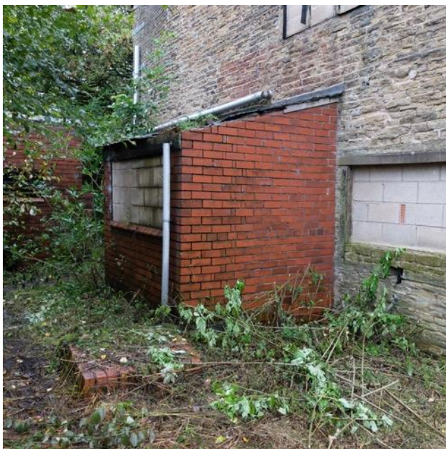
Photo. Brick porch, poor quality
