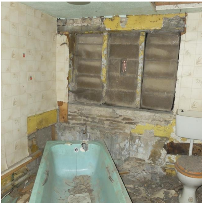
Photo. Added and damaged plaster east gable. Room F.08
