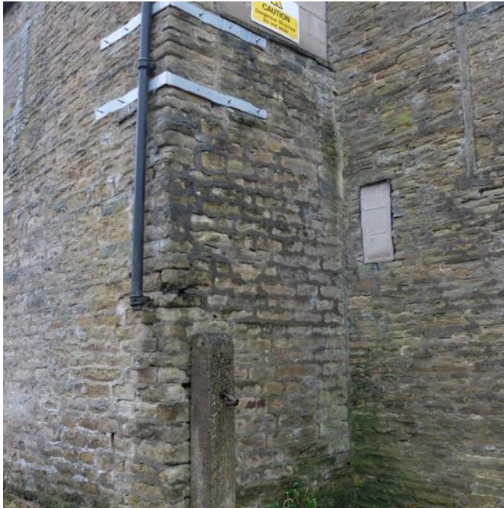
Photo. Eroded stone
