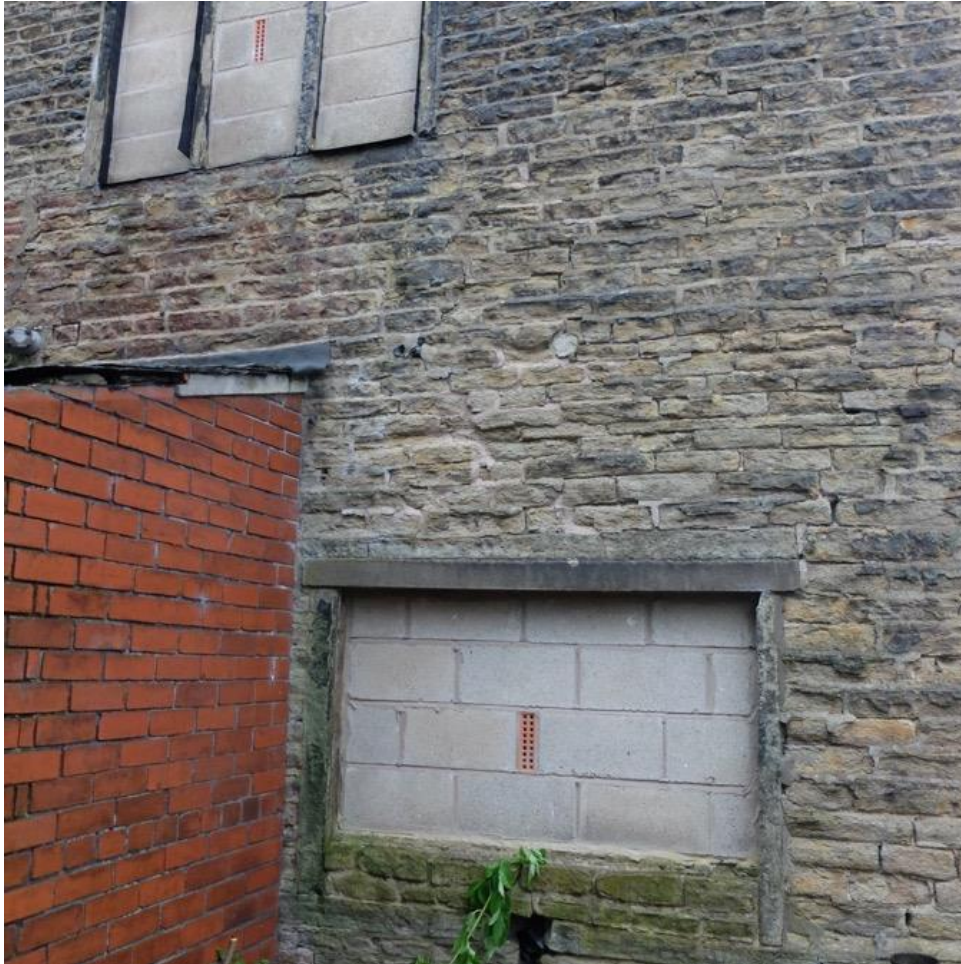
Photo. Cracking between ground and first floor windows.
