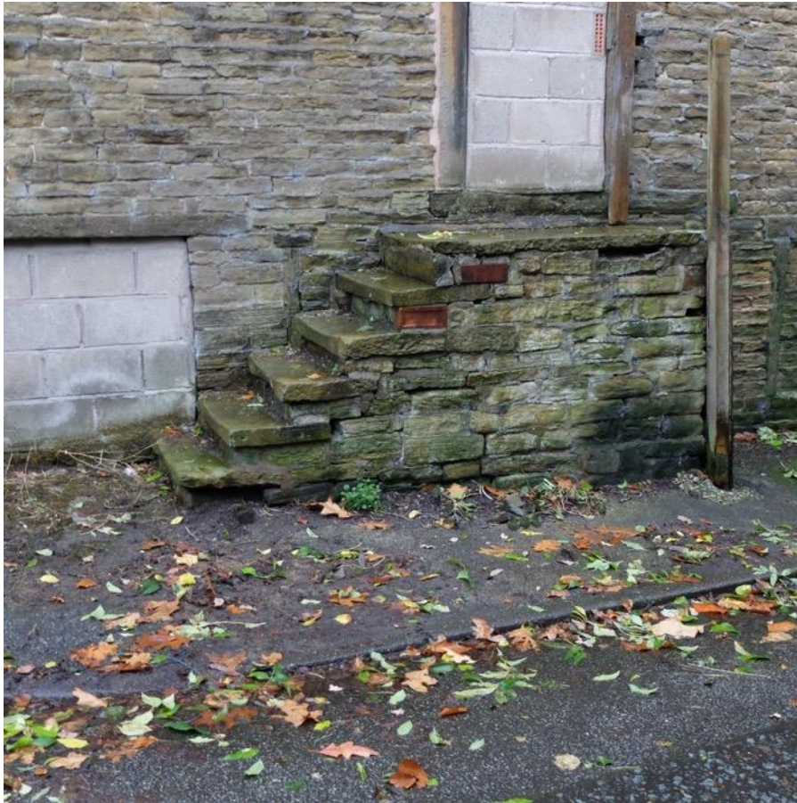
Photo. Later stone steps to gable door will require rebuilding
