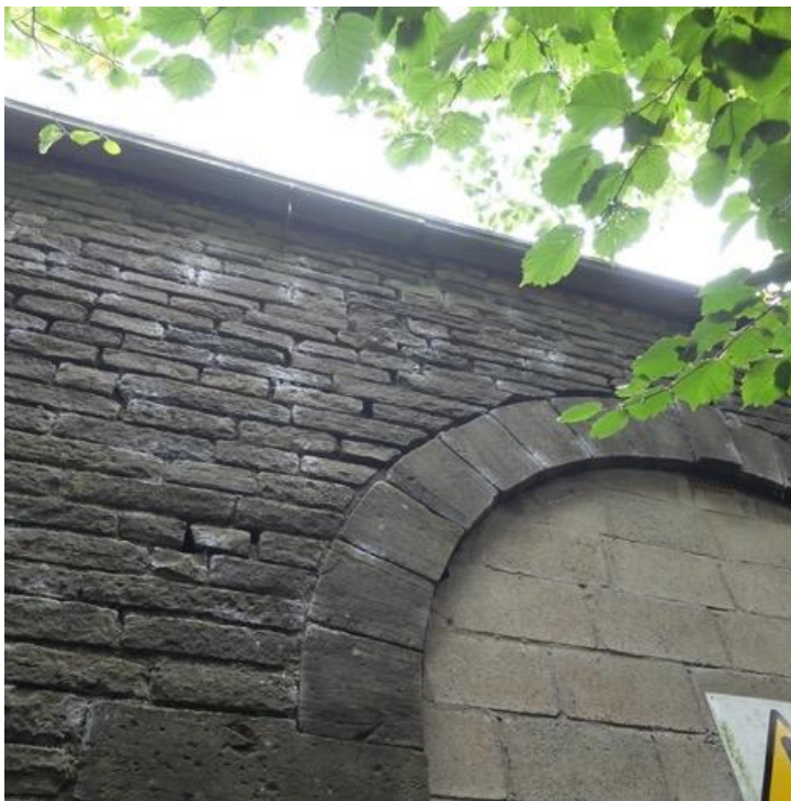
Photo. Mortar was away by leaks
