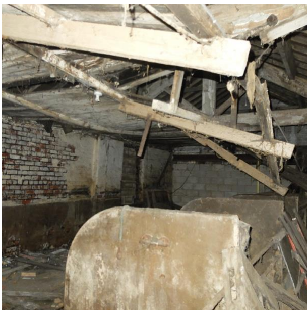
Photo. Collapse of roof structure to single storey building abutting barn
