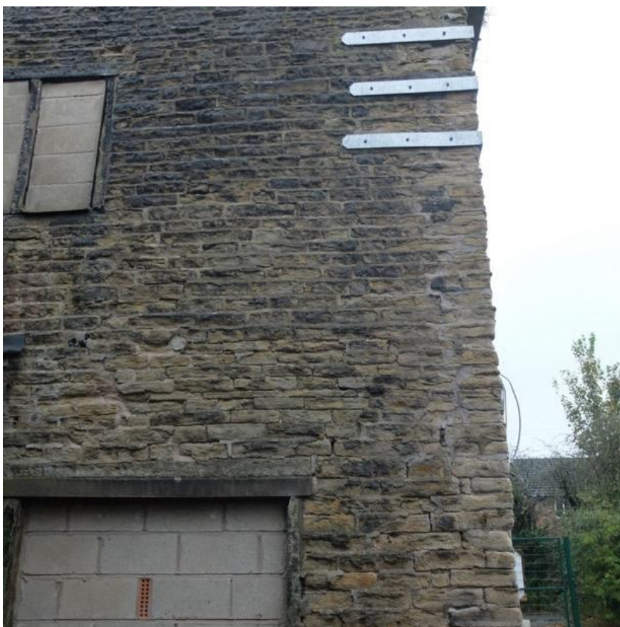
Photo. Frost damaged and eroded stone.
