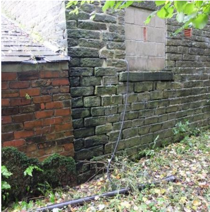
Photo. Loose brickwork at ground level
