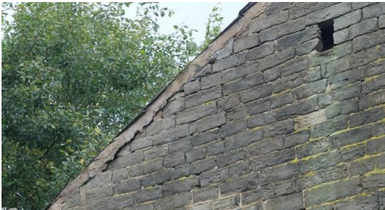
Photo. Loose cement verge pointing
