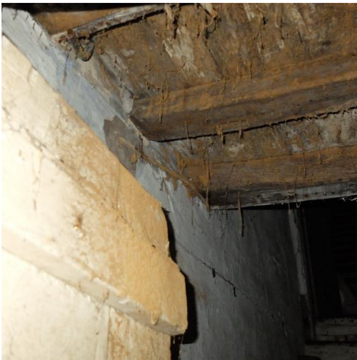
Photo. Decay to joists and boards which support York stone floor above, Room B1
