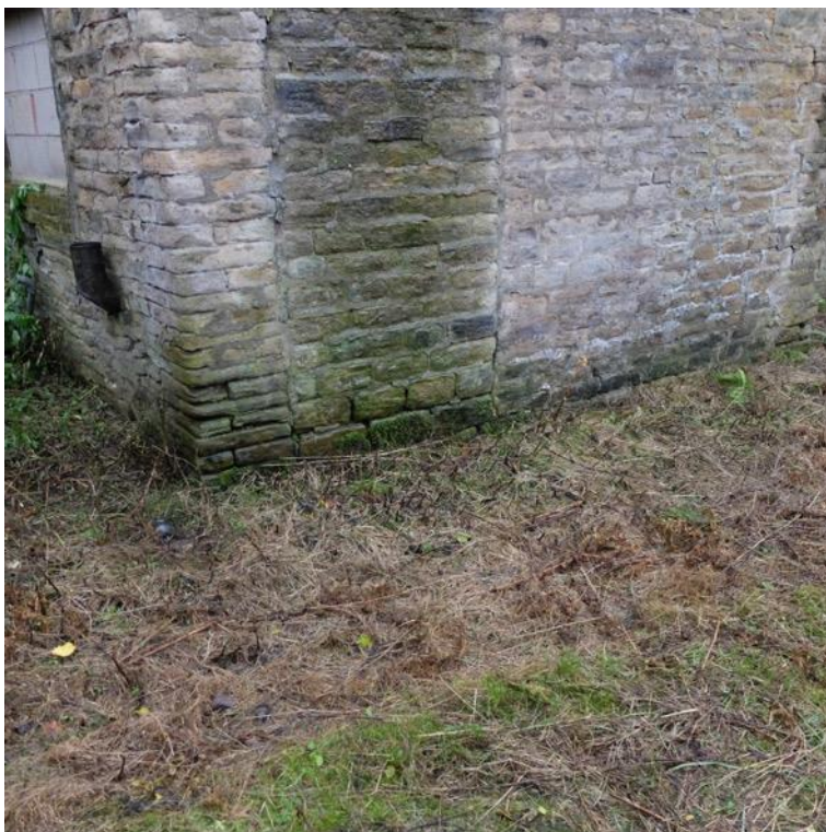
Photo. Crack along vertical joints between wall and infill.
