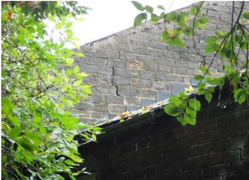
Photo. Movement extends up to roof level
