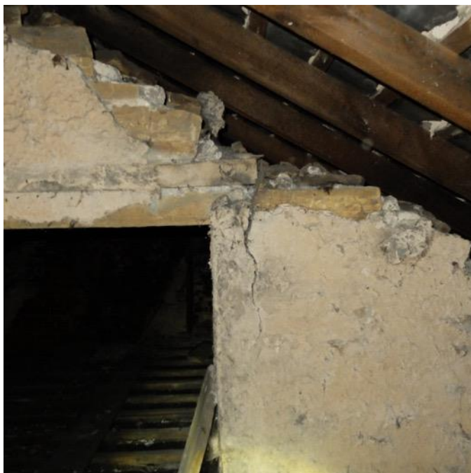
Photo. Crack around lintel to opening between roof spaces R1 and R2
