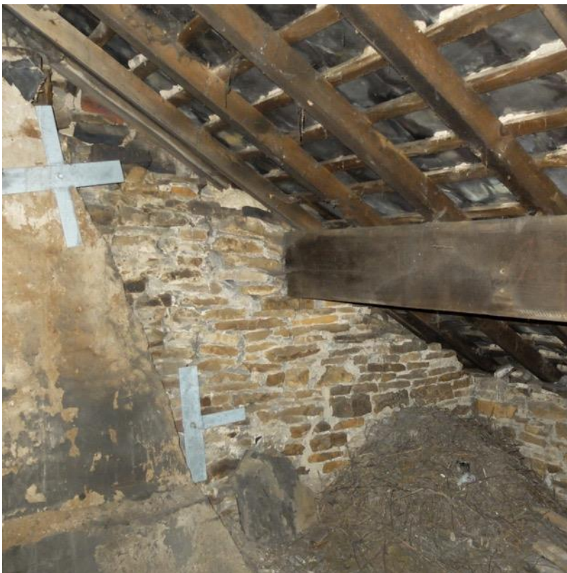
Photo. Tie plates and bulge in outer leaf behind this section.
