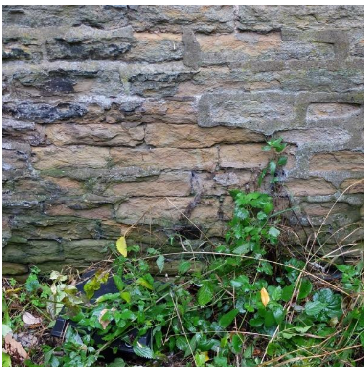
Photo. Corroded and frost damaged stone beyond repair.
