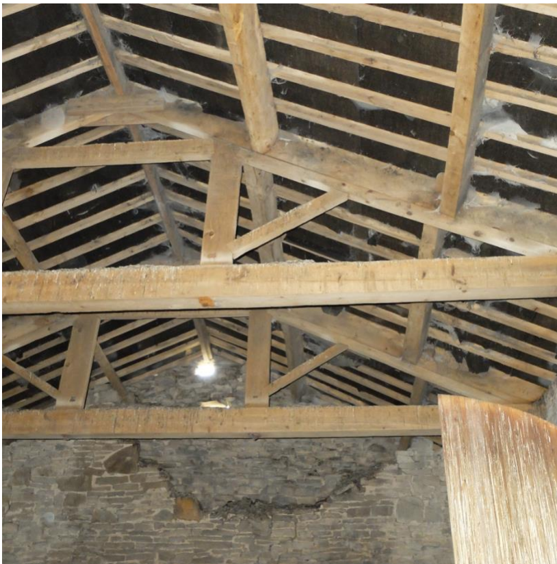
Photo. Collapse of inner leaf to gable.
