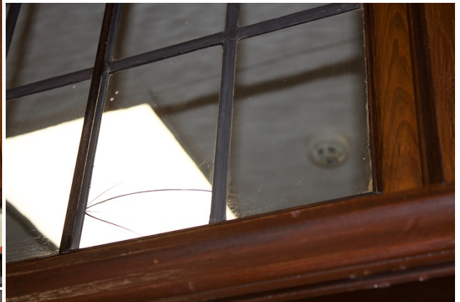
Damaged pane to internal window
