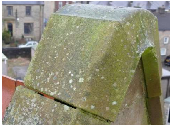
The apex capping stone is de-bonded and remains in position by gravity. It can easily be lifted off the gable. An open joint is visible above.
