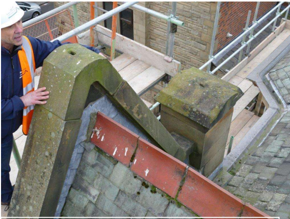
The top panel of the entrance gable can be rocked on its bed joint, three metres below at the head of the stair window.
