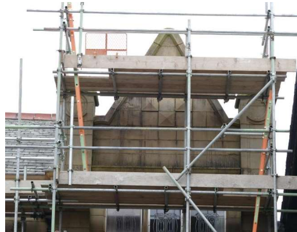
The upper section of the gable is loose and is flanked by two piers with raised heads. The central panel appears to be un-bonded and the right hand pier has displaced to the south. The stonework of the pier is also displaced below.
