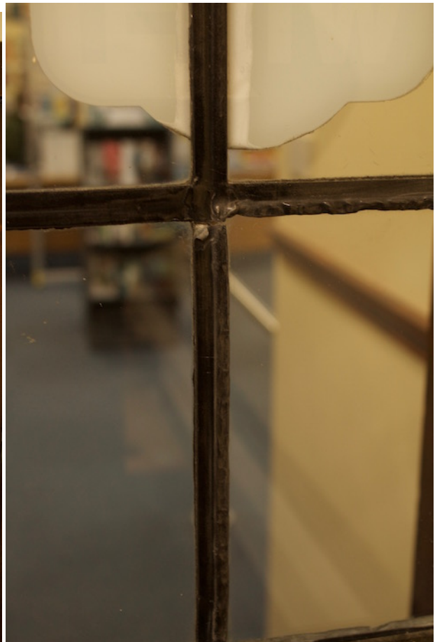
Loose lead in door panel
