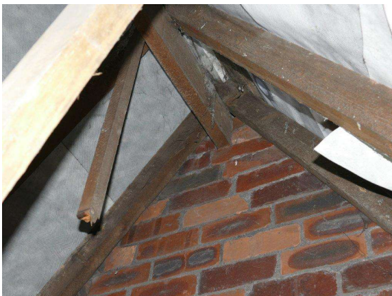
Roof spars offer little real support to the gable and appear not to be strapped or tied to the gable in any way..
