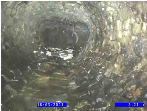
UpstreamX_58999eb5-f369-49fd-aa40-196d5b0d55b6_20210325_090653_387.jpg, 00:02:26, 5.21 m Infiltration, dripping from 11 o'clock to 1 o'clock
