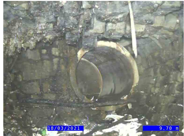
UpstreamX_978c7c51-c7b3-4809-a74b-be8b13f5dae1_20210325_090812_218.jpg, 00:04:18, 9.70 m Survey abandoned, Due to obstructions in pipe
