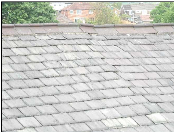
Figure 16: Signs of movement in the roof of Building 1.
