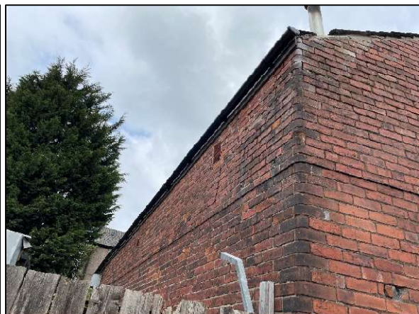
Figure 21: The brickwork and fascia board of Building 3.
