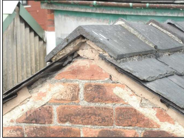
Figure 15: Voids in the verge to the east of Building 1.
