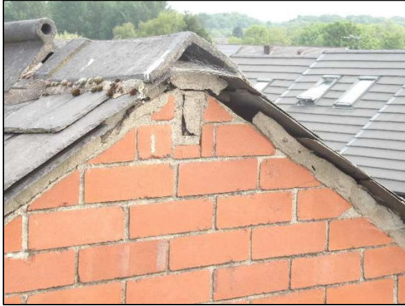
Figure 14: Voids in the verge to the south of Building 1.
