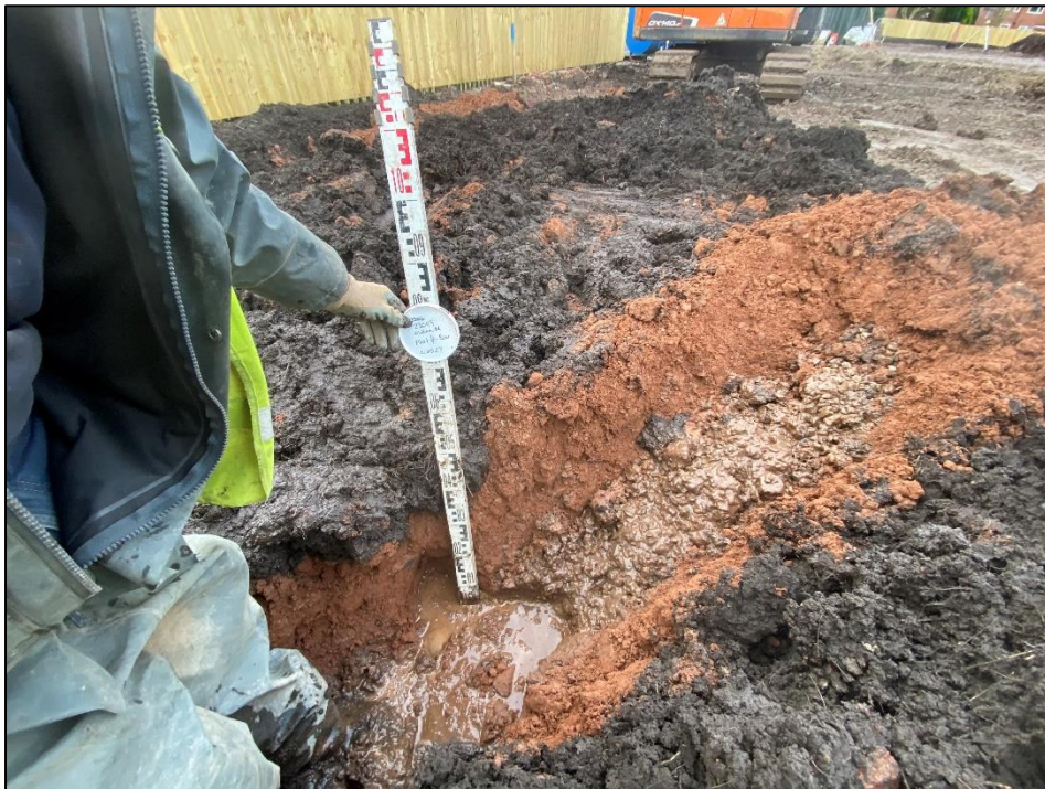
View of Plot 4 rear garden excavated to a depth of 0.60m, perched water ingress within the sand subsoil material.
