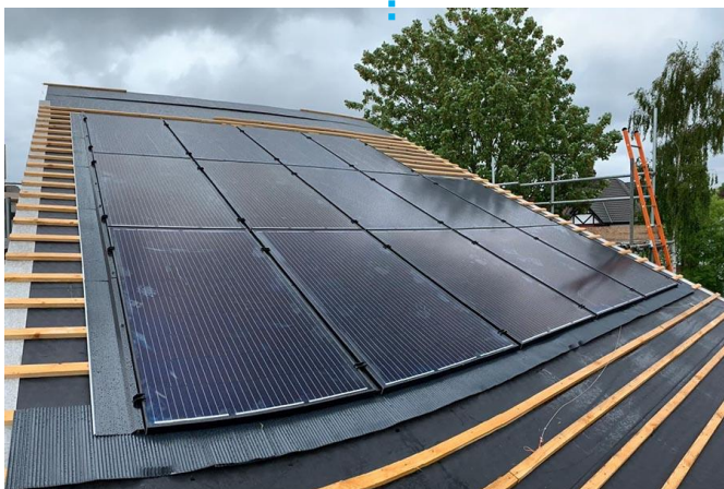
integrated PV panels
