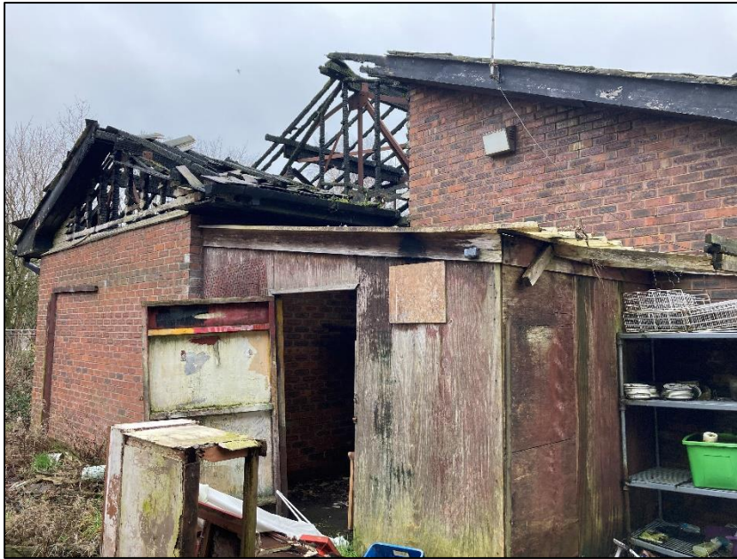
Photograph 9 showing the fire damaged eastern extension
