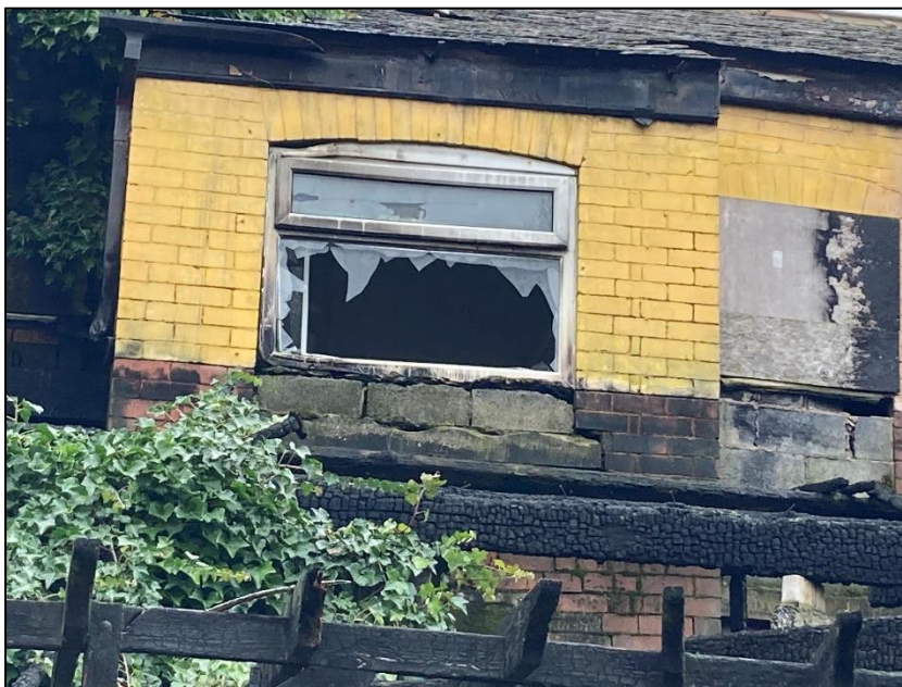
Photograph 10 showing the fire damaged windows at the rear of the property
