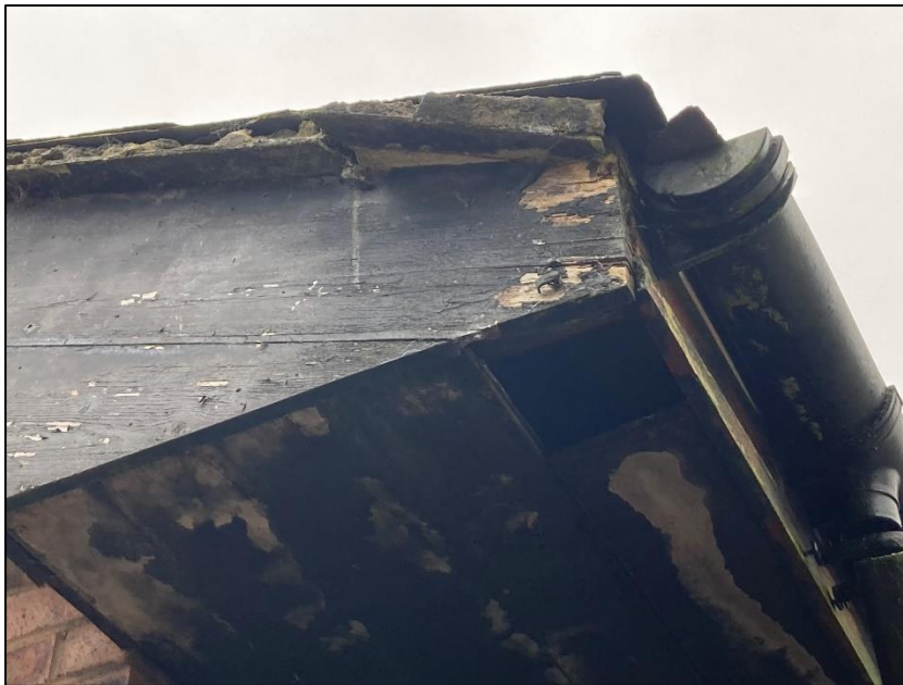
Photograph 11 showing a potential access point within the soffit boards
