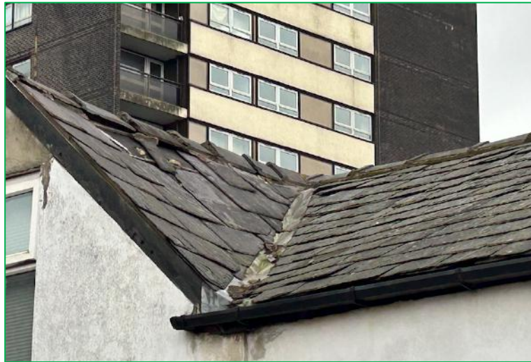
Showing raised, slipped and missing tiles
