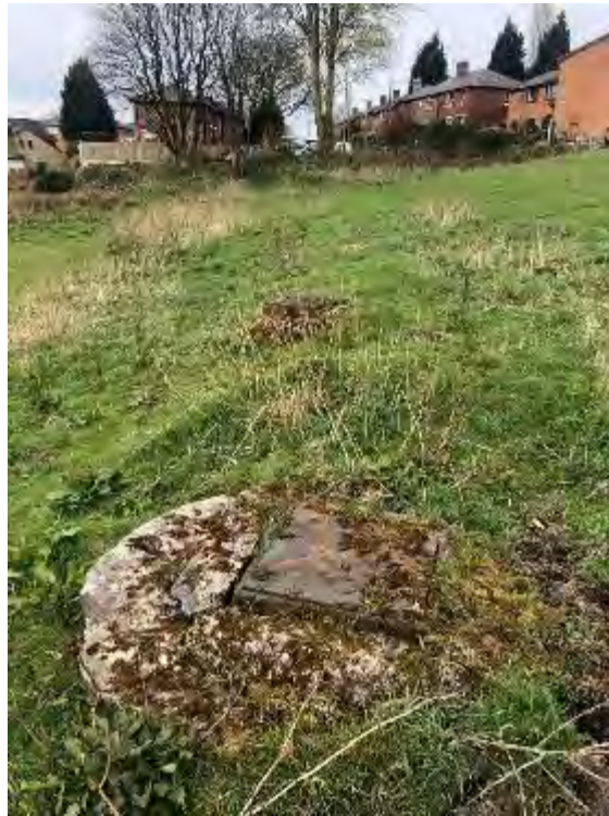
PLATE 7 RAISED MANHOLE COVERS – SOUTHWEST
