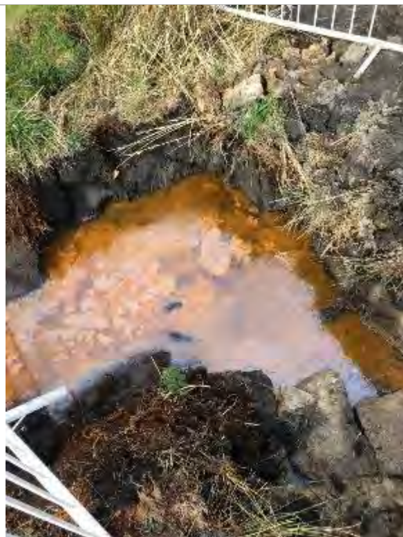
PLATE 2 ORANGE STAINING IN STAGNANT WATER
