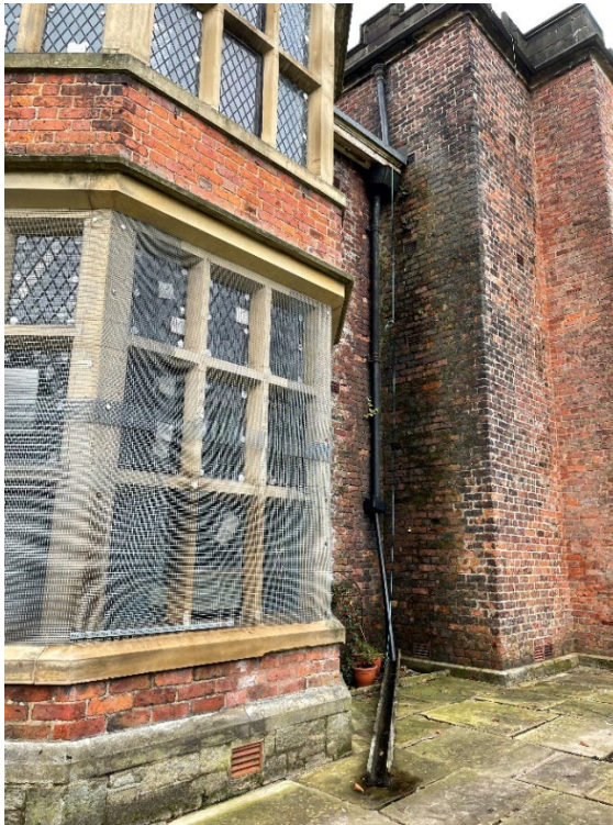
Figure 02 Rainwater pipe failure affecting the brickwork to the south-east of the Hall.
