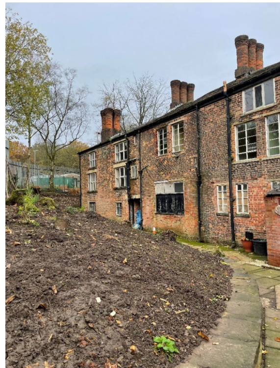
Figure 03 West wing of the building which is in a very unsafe condition structurally.
