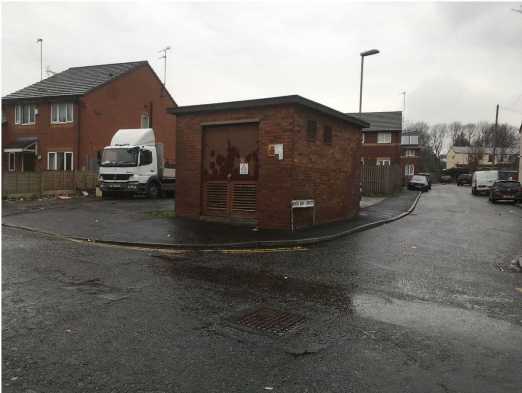
Photograph 5 – Electric substation Block C.
