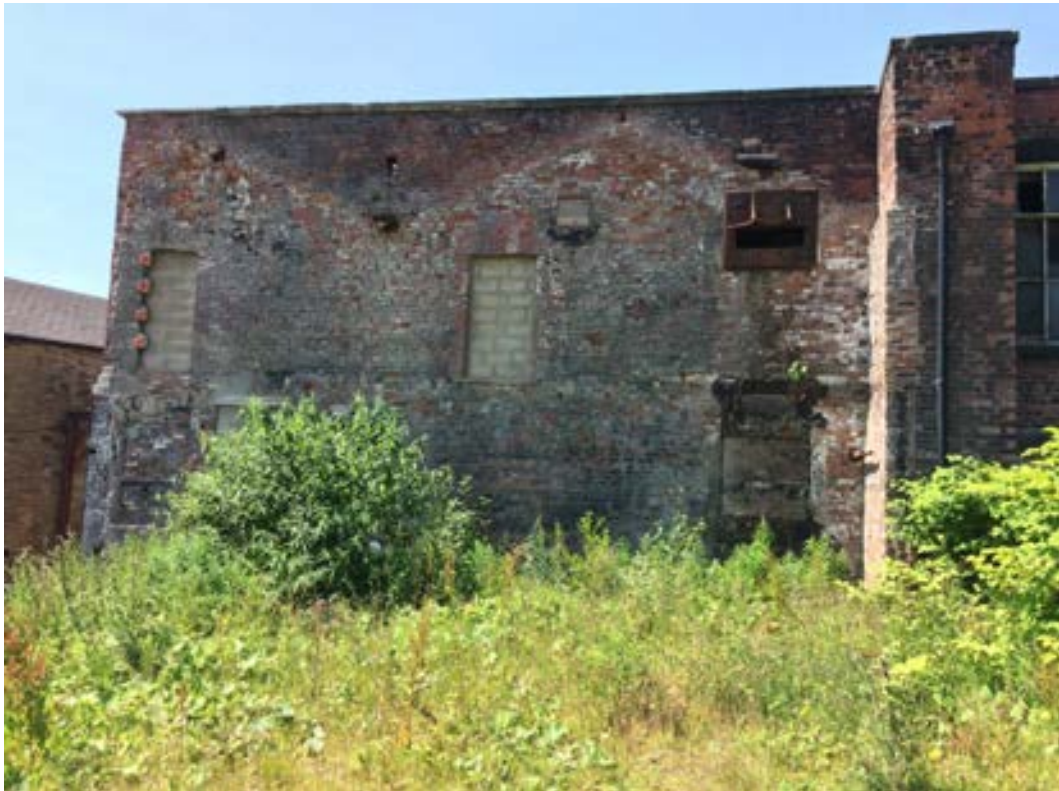
Plate 30: Evidence of the c. 1800 weaving shed on the north-east facing elevation of the extant mid-19th century range.
