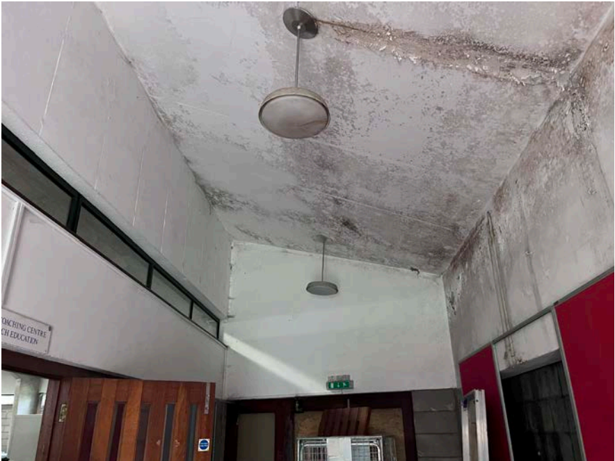
WATER DAMAGED CEILING TO NARTHEX
