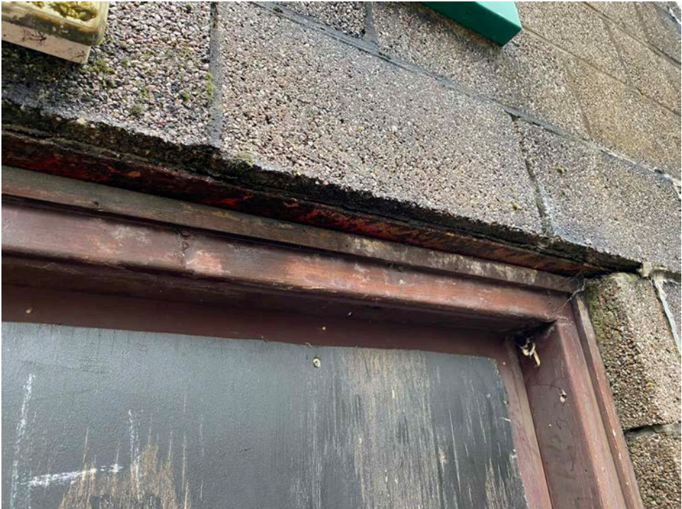
CORRODED LINTEL ABOVE MAIN ENTRANCE DOORS
