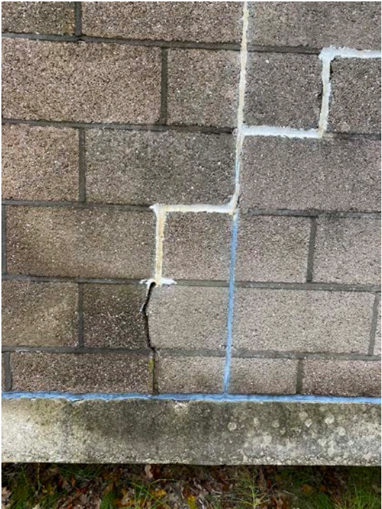
AREA OF INAPPROPRIATE POINTING
