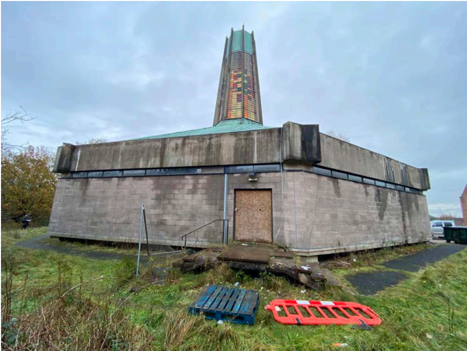
REAR FACADE SHOWING AREAS OF DAMAGED CONCRETE
