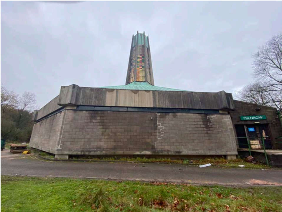
FACADE SHOWING AREAS OF STAINING AND LATER INAPPROPRIATE POINTING
