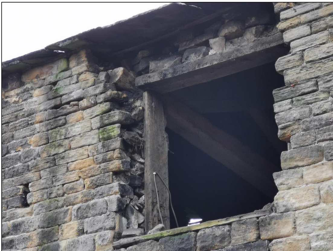
Plate 10 - Evidence of a cavity inside the stone fabric of the barn
