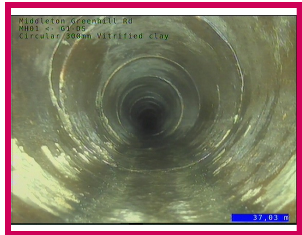
2, 00:02:56, 37.03 m Crack, circumferential from 9 o'clock to 1 o'clock
