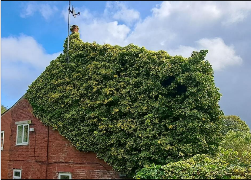
Photograph 11 showing Ivy obscuring a portion of external masonry
