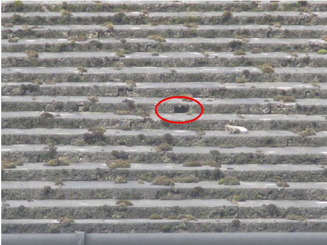
Photograph 7 – Examples of cracks and gaps in tiling across the roofs of Buildings 1 & 2.
