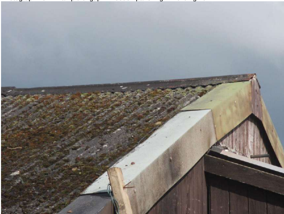
Photograph 14 – Example of gaps under loose fitting metal sheeting covering gable end on Building 10.
