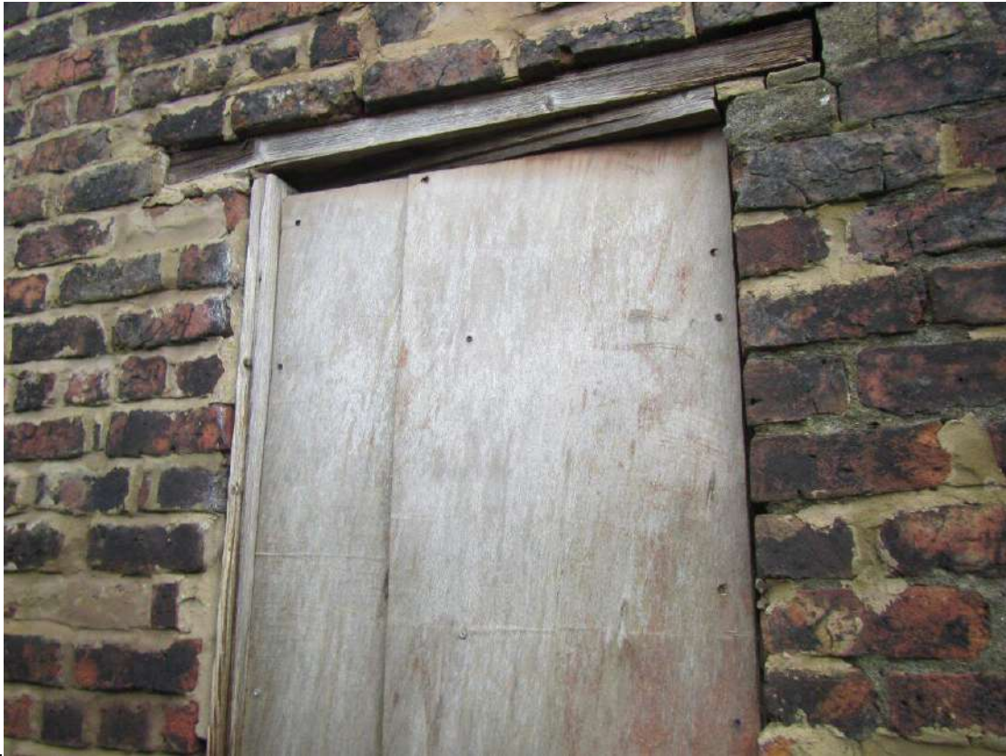
Photograph 11 – Example of gap around the windowframes in Building 2.
