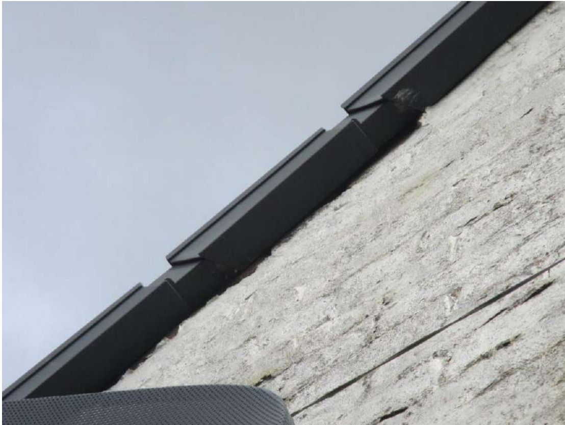
Photograph 9 – Covering of roofline on eastern gable end of Building 1, showing PRFs created by loose covering.
