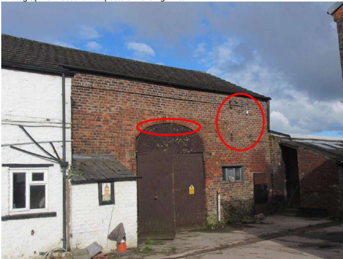
Photograph 4 – Northern aspect of Building 2, ventilation gaps can be seen on the top right section of wall (present on all aspects). Additionally a large gap is present between the door and the lintel.
