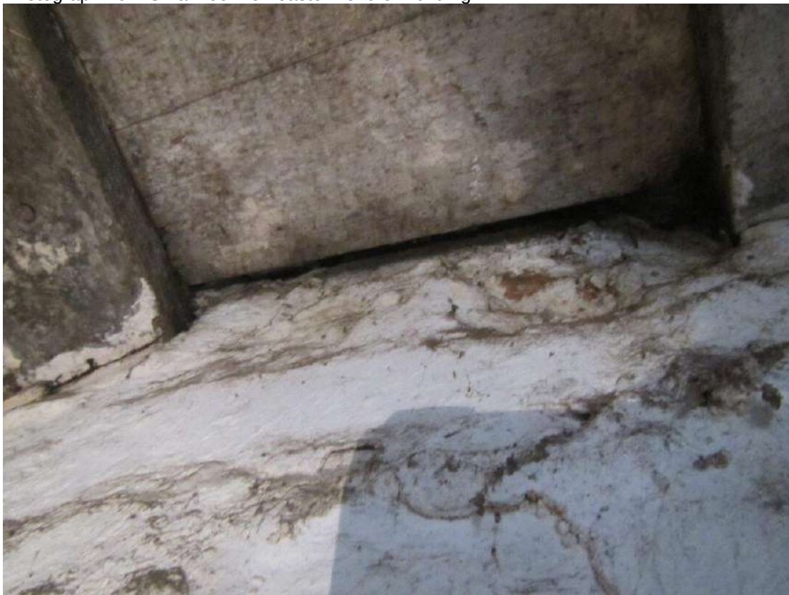
Photograph 30 – Gaps between ceiling pannels within small room on eastern end of Building 2.
