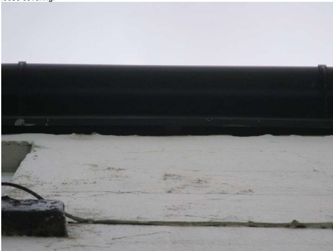
Photograph 10 – Gap between fascia and wall plate on southern aspect of Building 1.
