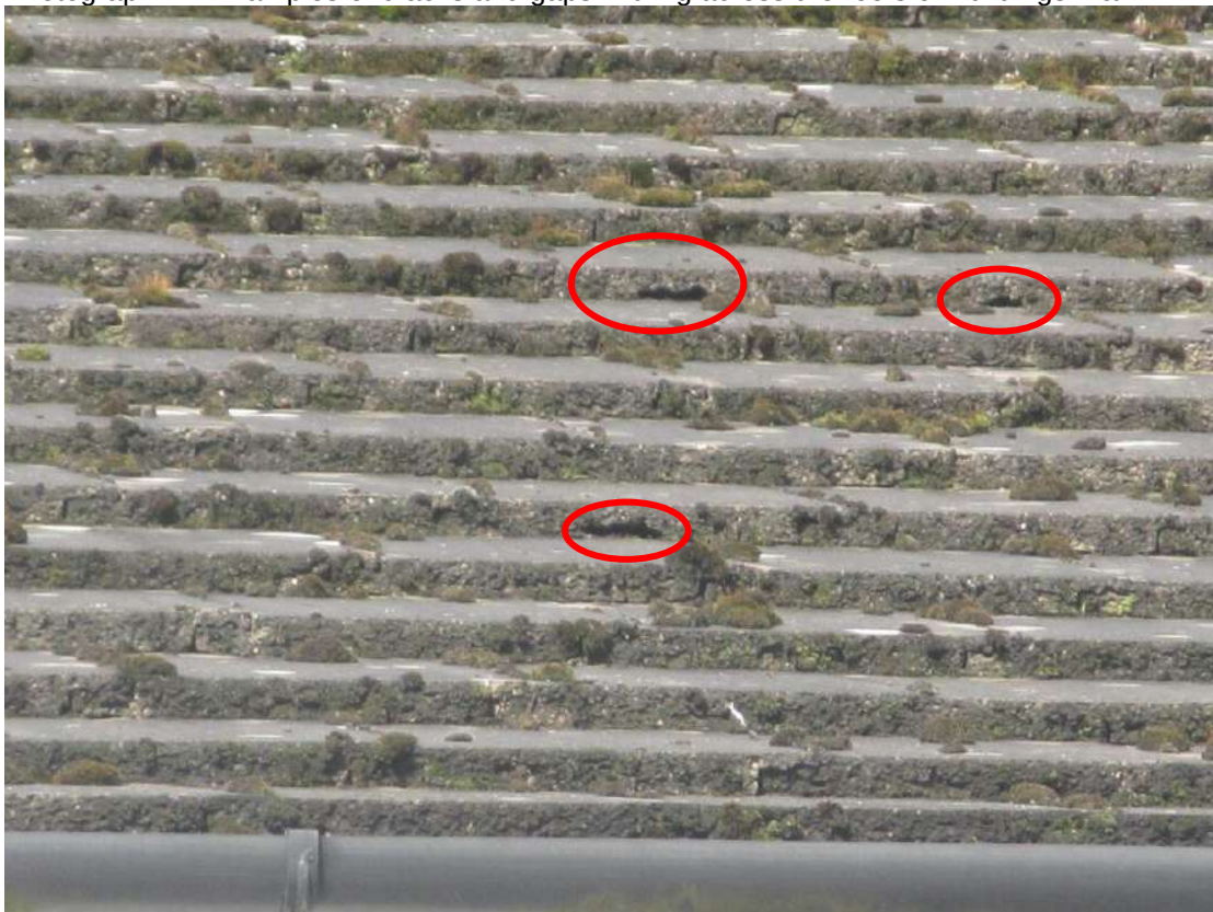
Photograph 8 – Examples of cracks and gaps in tiling across the roofs of Buildings 1 & 2.
