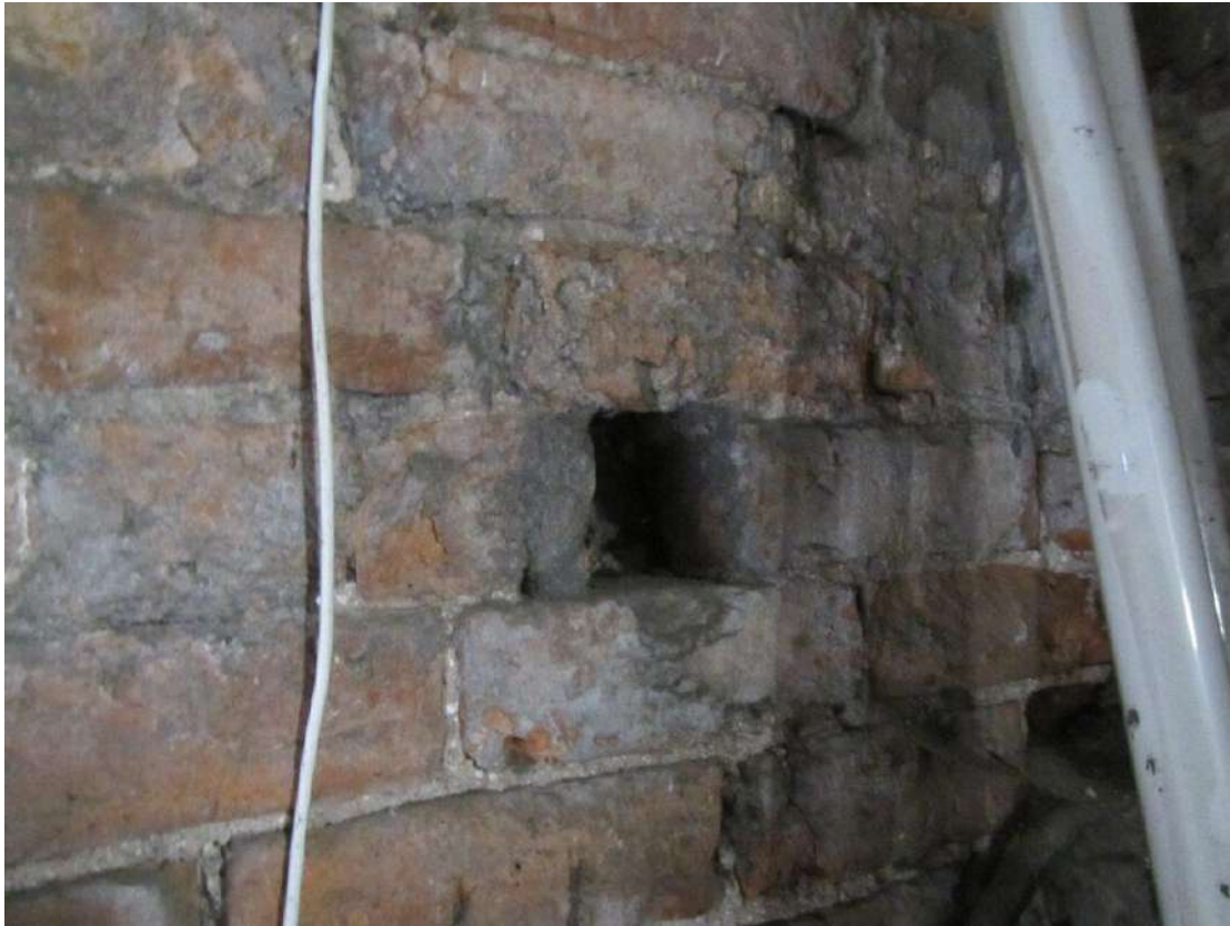
Photograph 25 – Example of gaps in the internal walls of Building 2.
