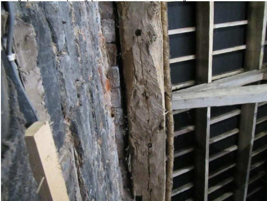
Photograph 26 – Example of gaps under exposed wall beam creating an ideal PRF inside Building 2.
