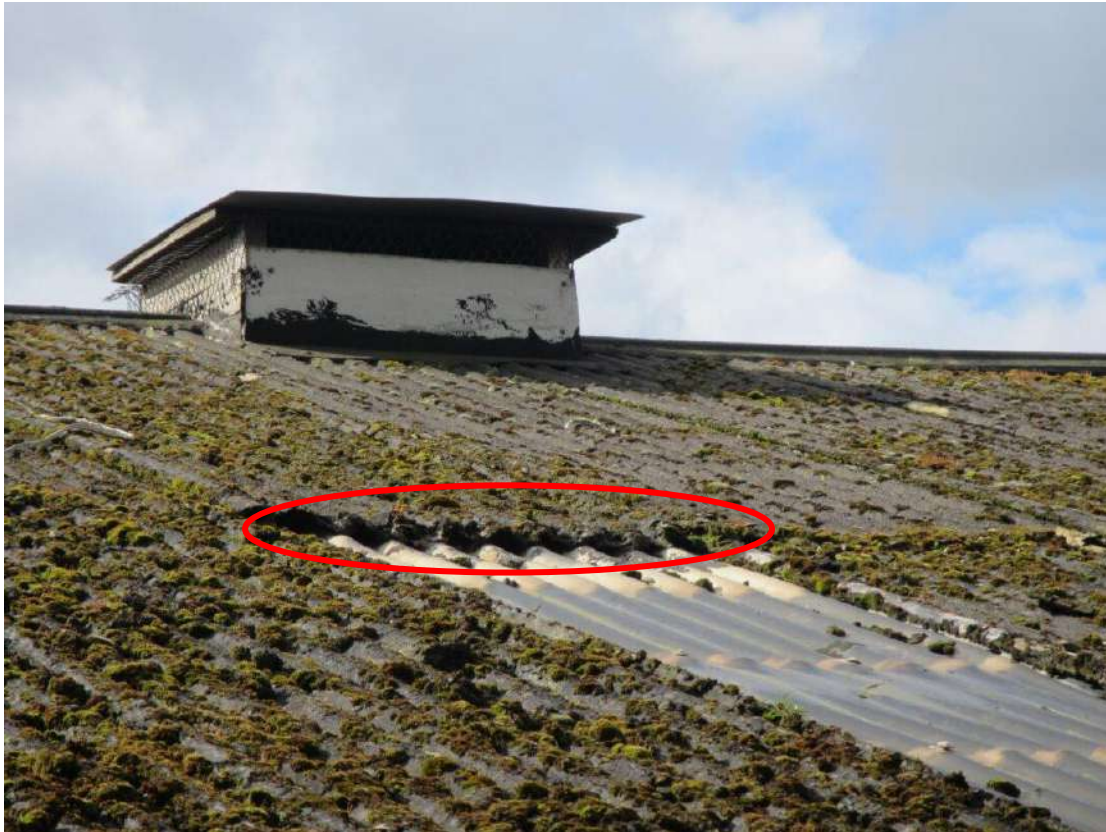
Photograph 15 – Example of gaps between asbestos sheeting on Building 10.
