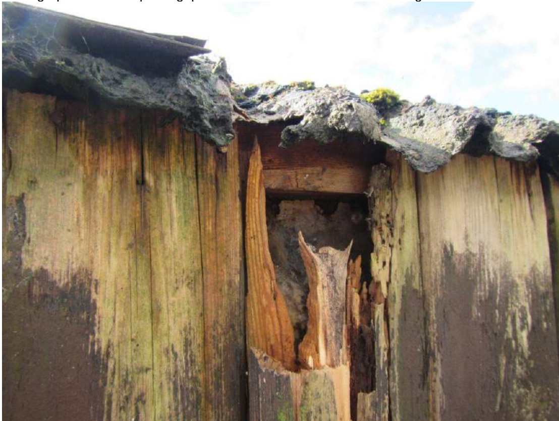
Photograph 12 – Example of gap in wooden panelling and gaps under the eaves in Building 10.
