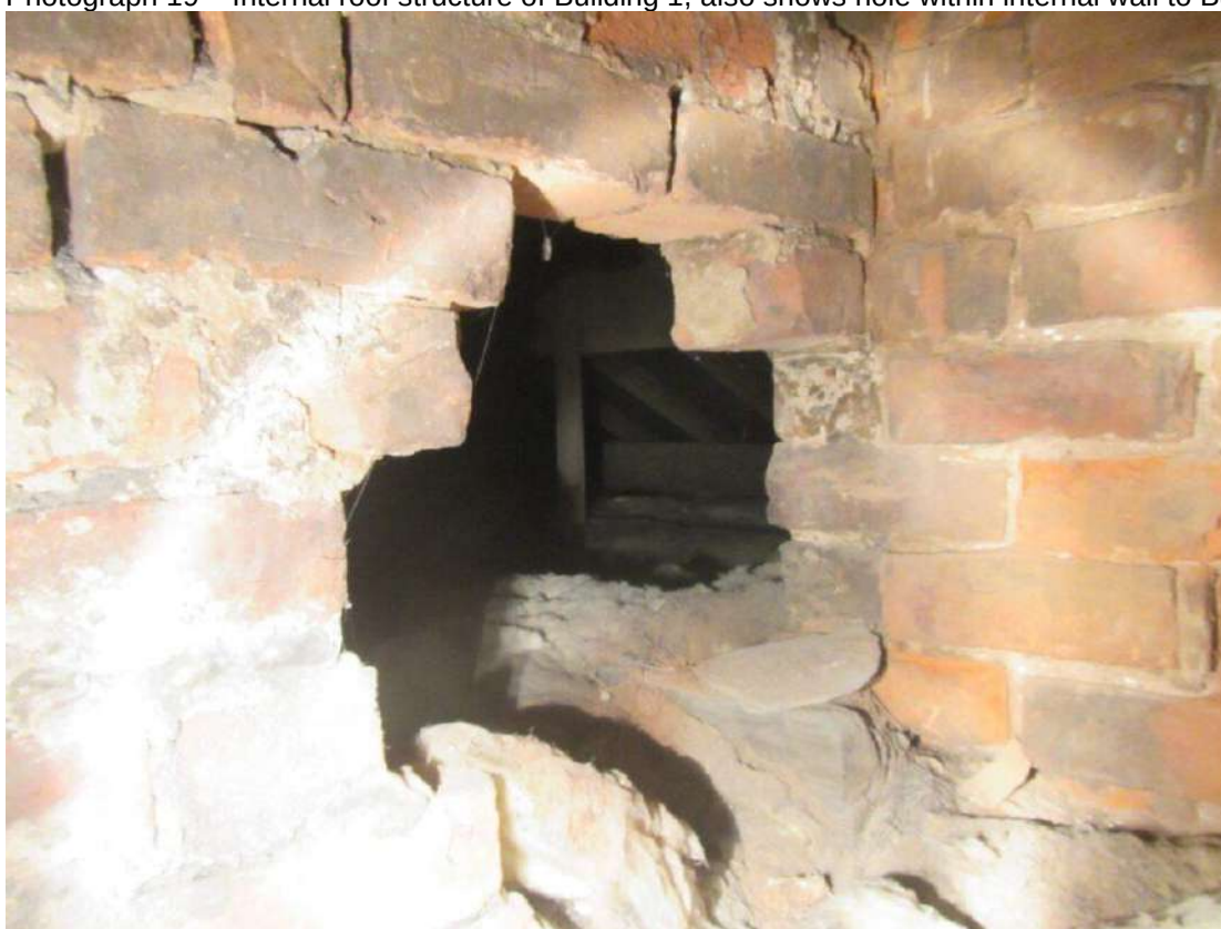
Photograph 20 – Gap in central internal wall withing roof void of Building 1.
