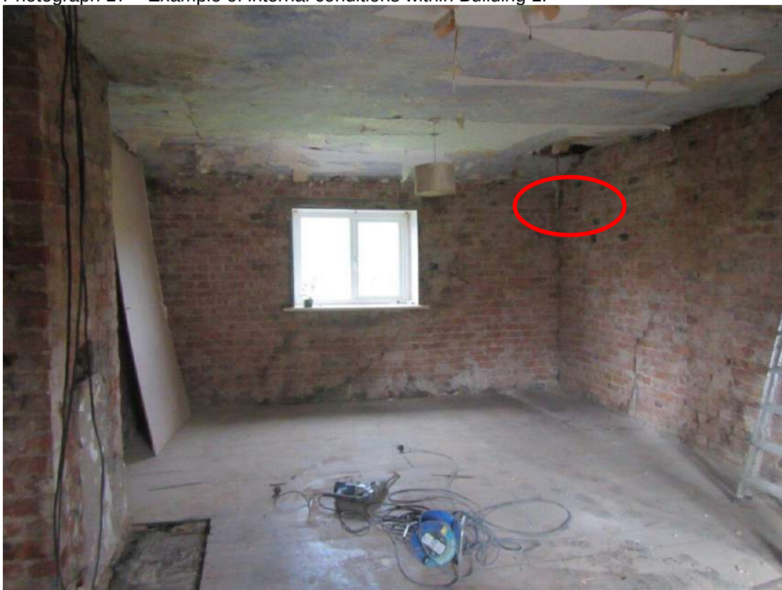
Photograph 18 – Example of internal conditions within Building 1 with section of collapsing ceiling.
