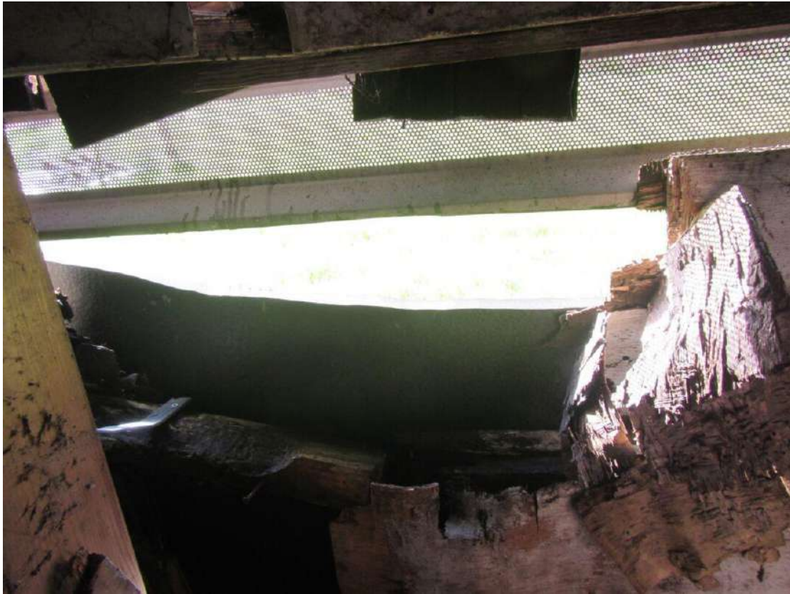
Photograph 13 – Example of gap in wooden panelling in Building 10.
