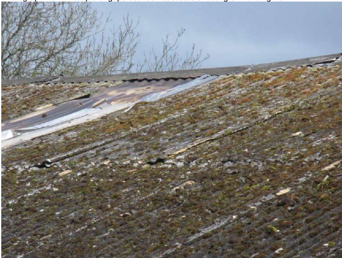
Photograph 16 – Example of gaps under ridgeline on Building 10.
