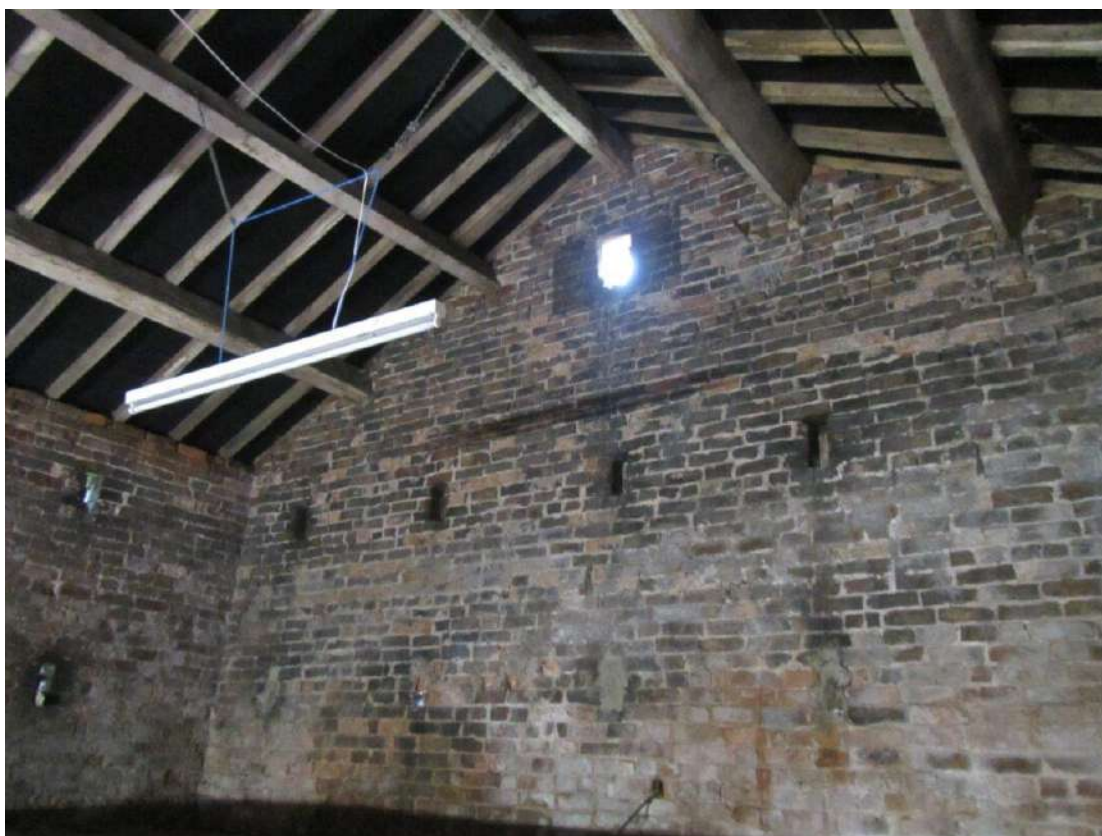
Photograph 23 – Interior conditions within Building 2, ventilation slits and open window near apex.
