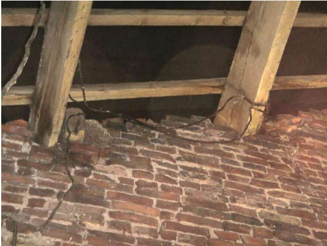
Photograph 27 – Example of gaps between brickwork and roof structure in Building 2.
