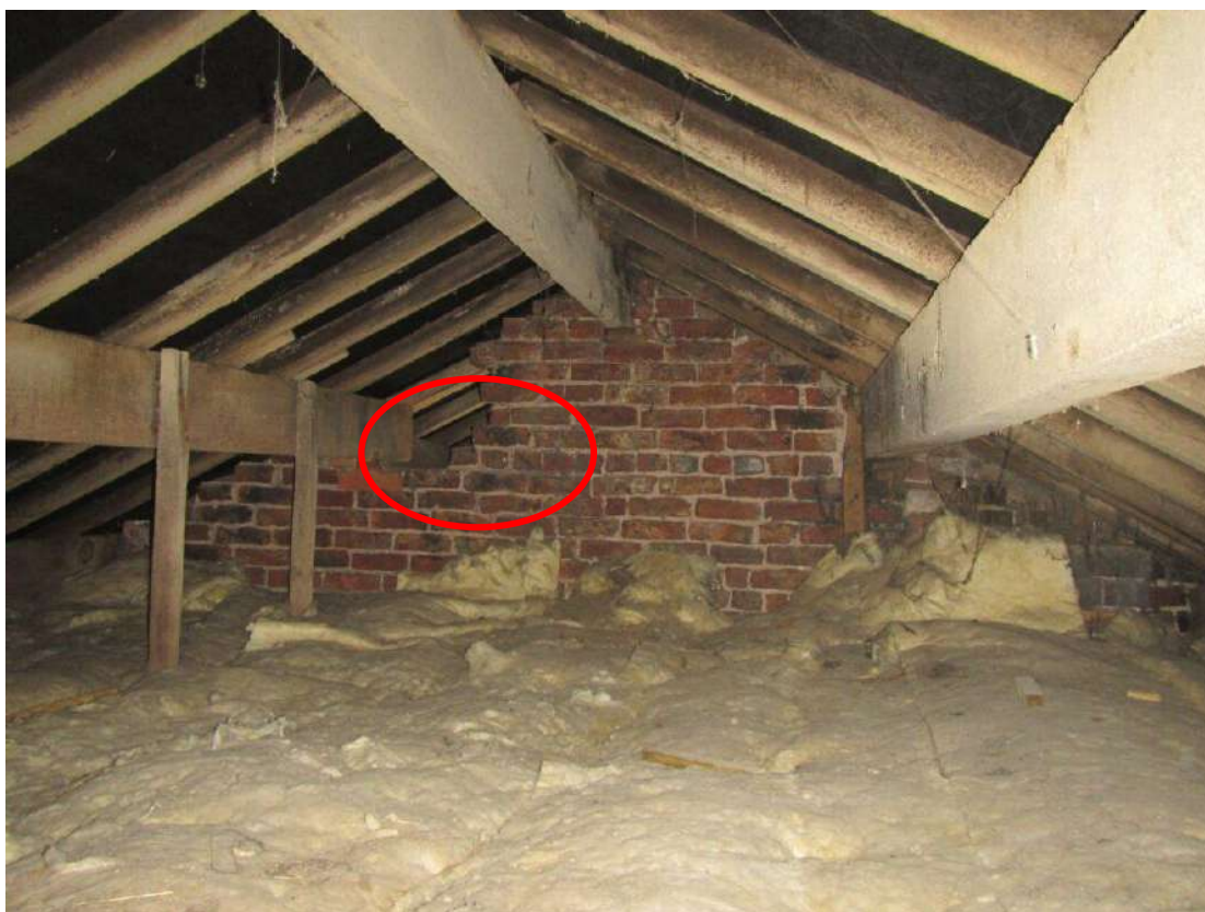
Photograph 19 – Internal roof structure of Building 1, also shows hole within internal wall to Building 2.
