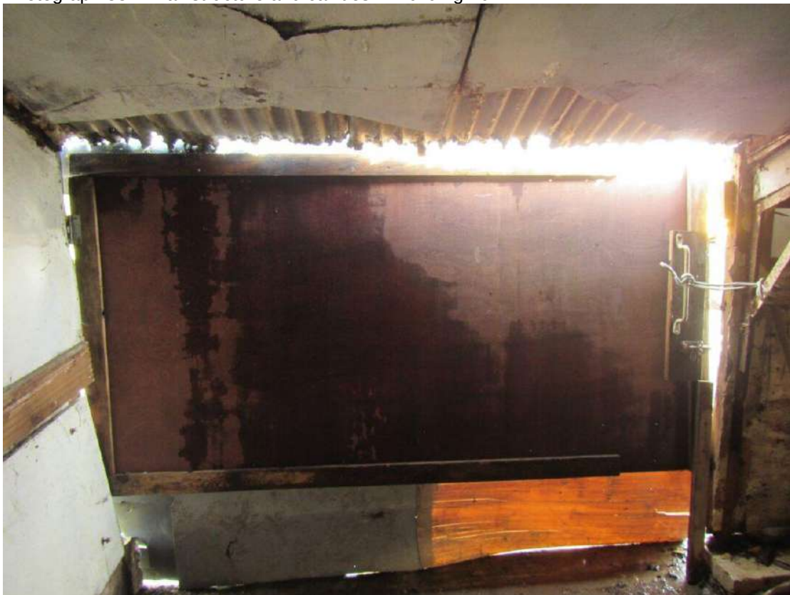
Photograph 34 – Example of gaps present in Building 10.
