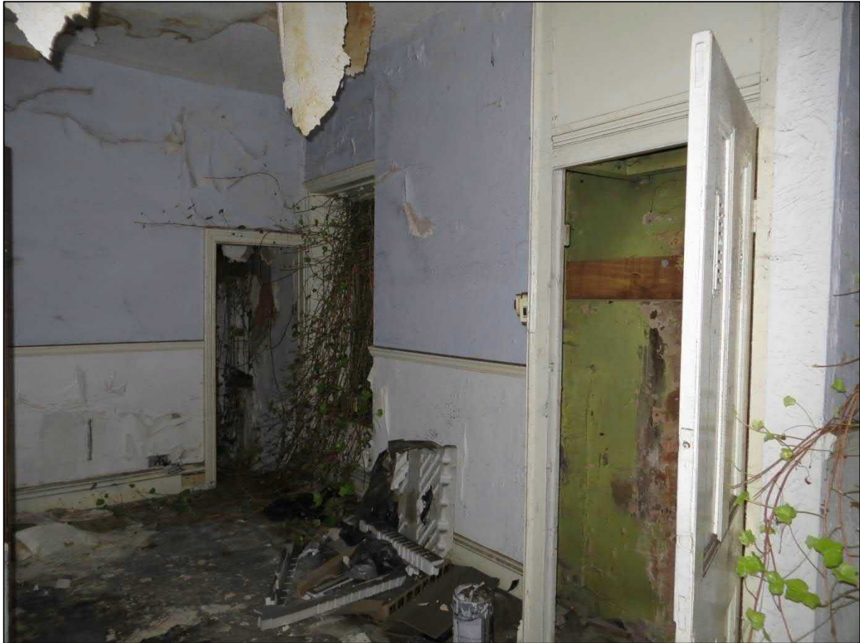
Figure 33: View from first floor interior looking towards the south external wall. Note the vegetation and collapsed ceiling.
