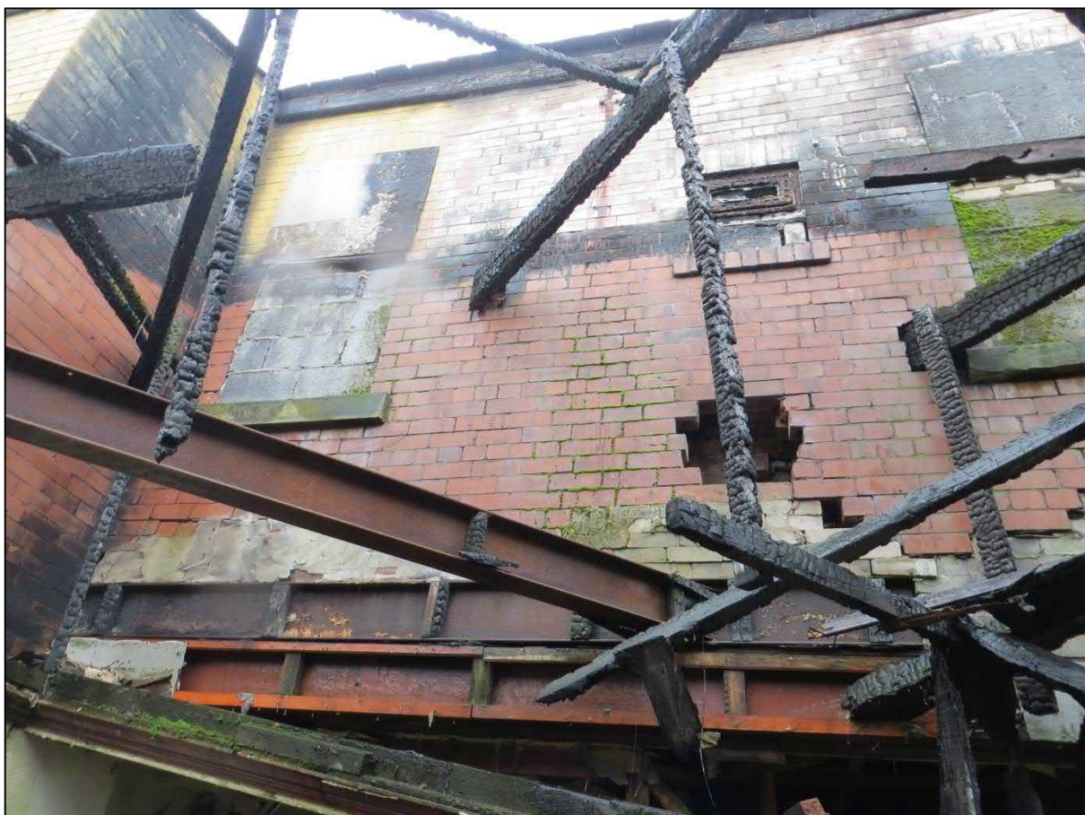
Figures 30 and 31: Views looking from ground floor within the fire damaged/collapsed extension towards the rear wall of the “original building”.
