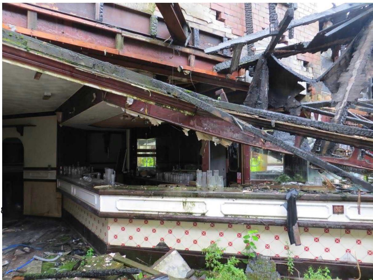
Figure 28: Ground floor interior. View looking from within the fire damaged/collapsed extension showing the opening in the "original building" rear wall.
