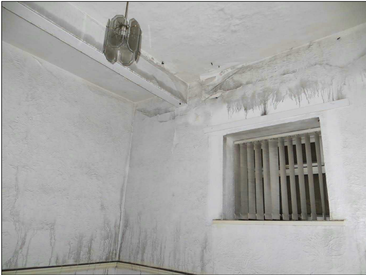
Figure 35: View of first floor interior with extensive water penetration. Note the low-quality contemporary windows.
