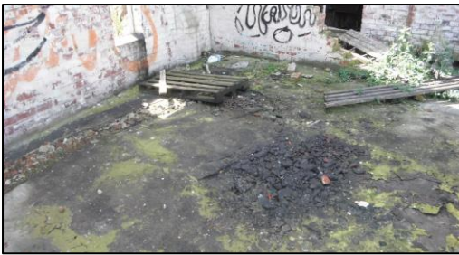
Potential spillages - putrid & minor H/C odours (Building 11)
