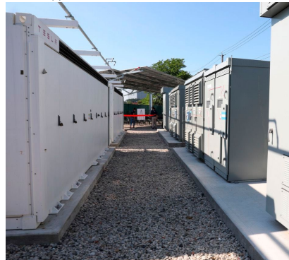
Battery storage units in greys
