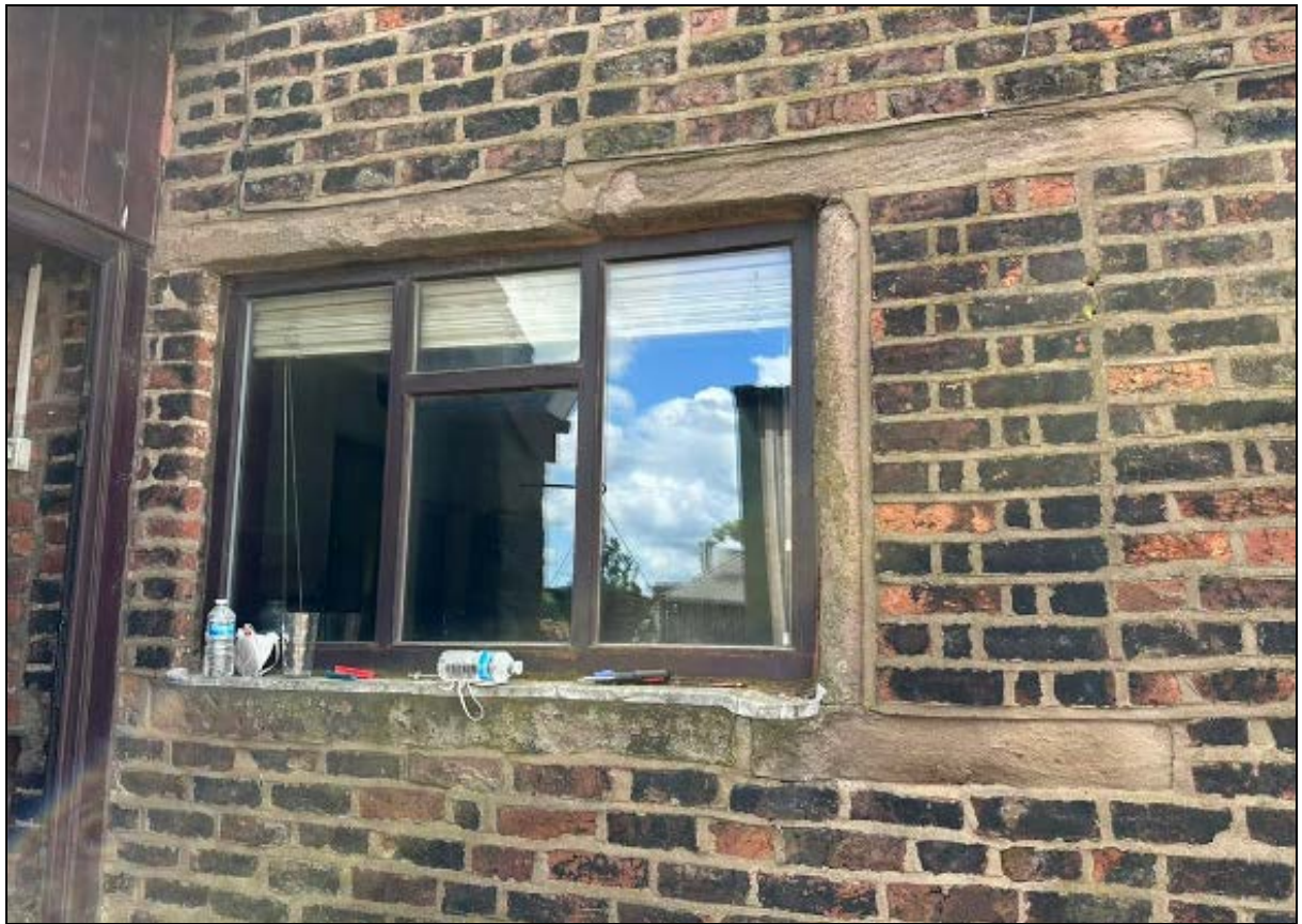
5. Kitchen window with mullion remaining
