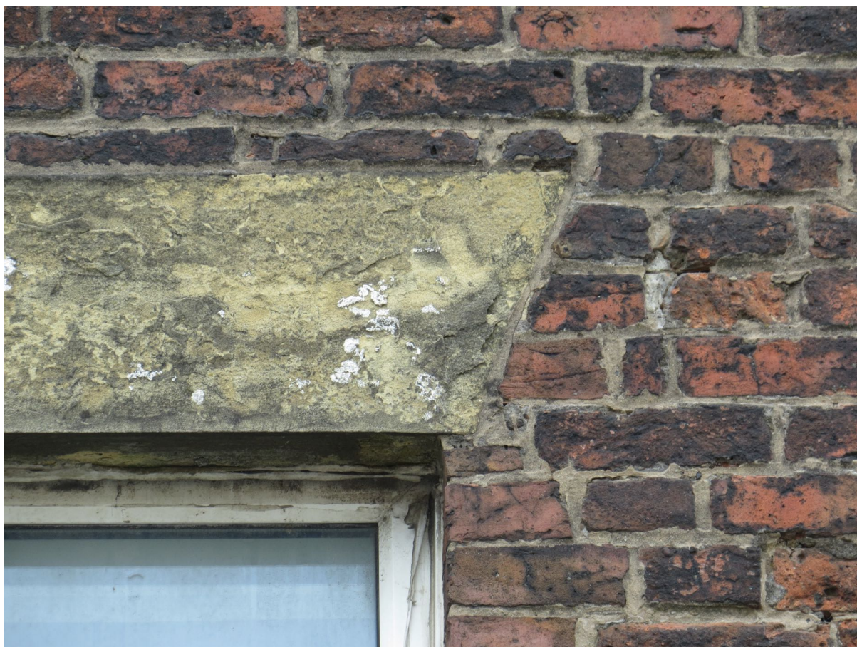
7 – Window and door frames are sealed into brickwork with no suitable gaps.
