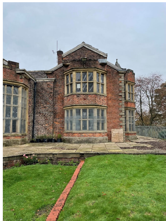
Figure 03 Degradation to the roofs throughout.
