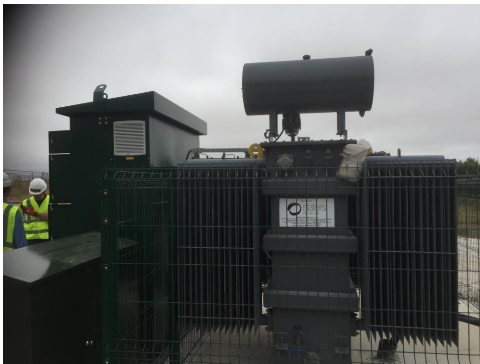
Figure 4 - Example Feeder Pillar Installation
