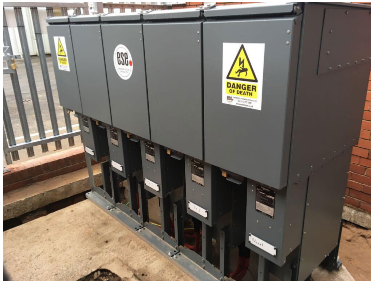
Figure 6 – Example External Switchboard
