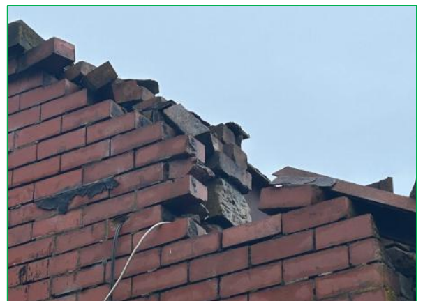
Cavities in the walls exposed to rain
