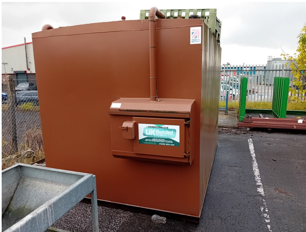
Photograph of fuel storage tank within machinery storage area in the west of the site. Taken looking southwest.
