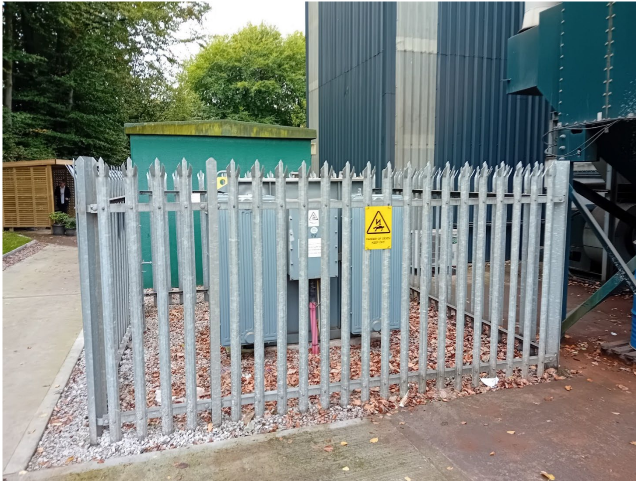
Photograph of electricity substation near southeast corner of main building. Taken looking south.
