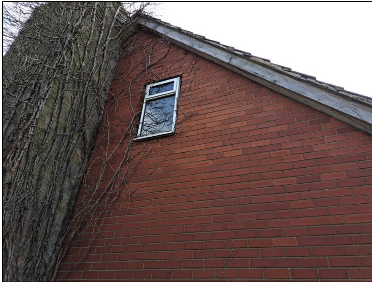
Photograph 4 showing gaps along the roof verge and around window
