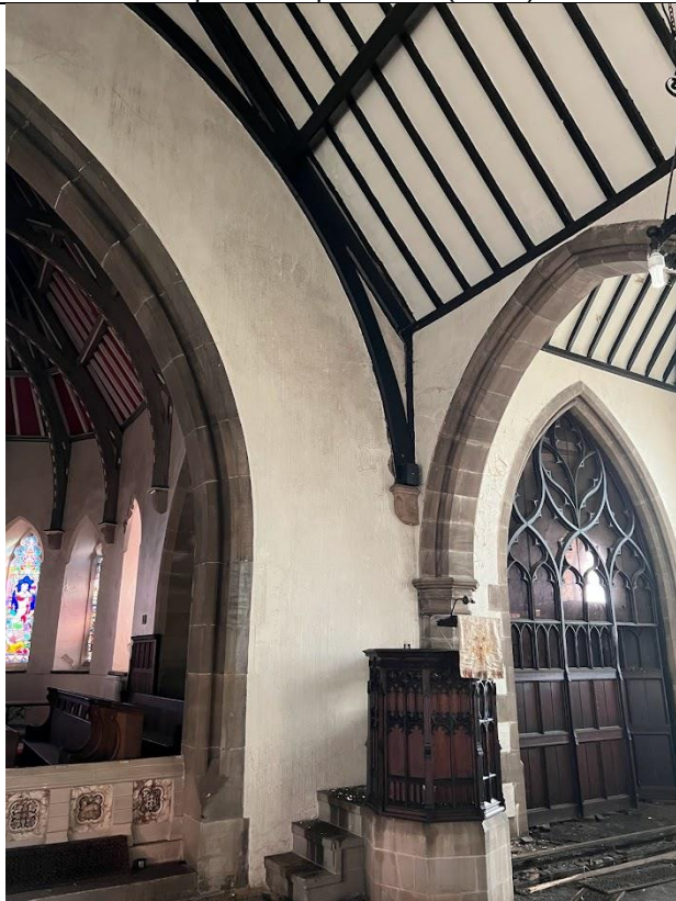
Roof truss and rafter requiring repairs (Item 2)
