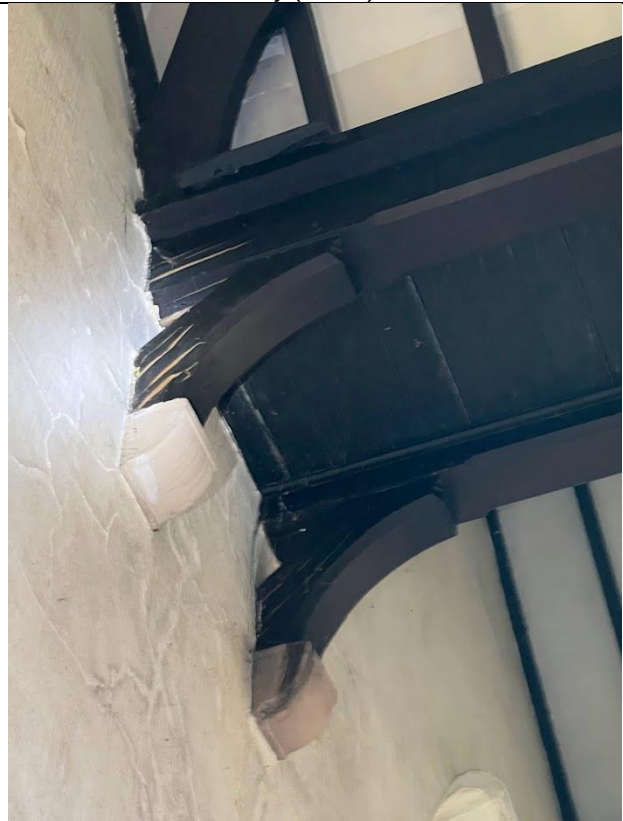
South Transept Valley timber decay (Item 6)
