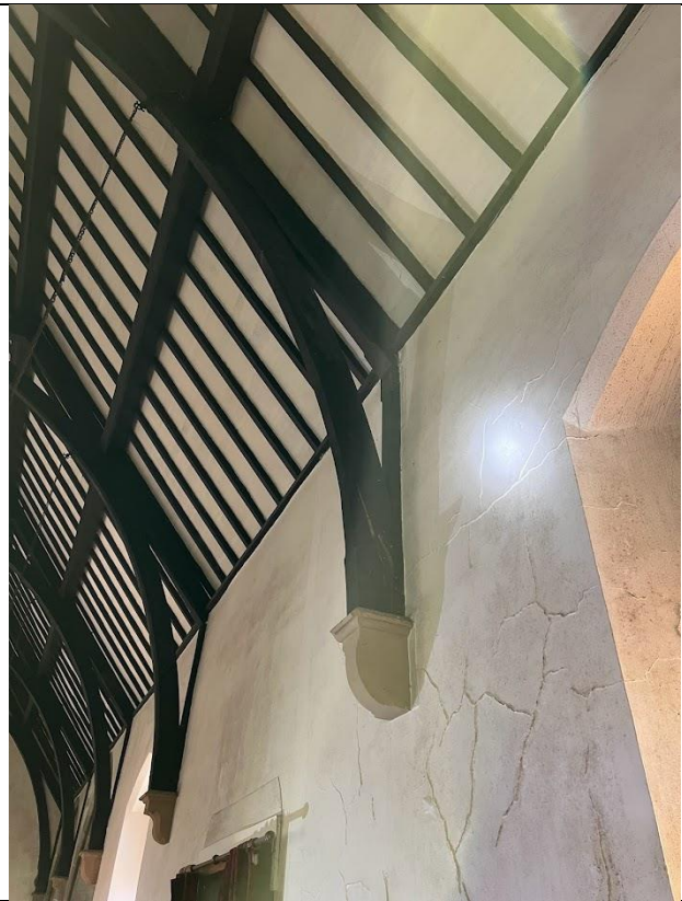
Further Nave Truss decay (Item 4)
