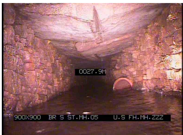
ZZZX_e4a6e72c-c616-483d-9fda-125620884cf1_20210427_1 12813_967.jpg, 00:02:36, 27.90 m Broken sewer from 11 o'clock to 1 o'clock, SLAB BROKEN
