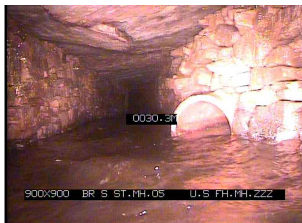
ZZZX_c4718e43-bf3e-4306-81df-7f17a0411a36_20210427_1 13023_517.jpg, 00:04:24, 30.30 m Connection, intruding at 3 o'clock, 225mm diameter, 200mm intruding
