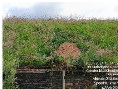
Fox den in embankment
