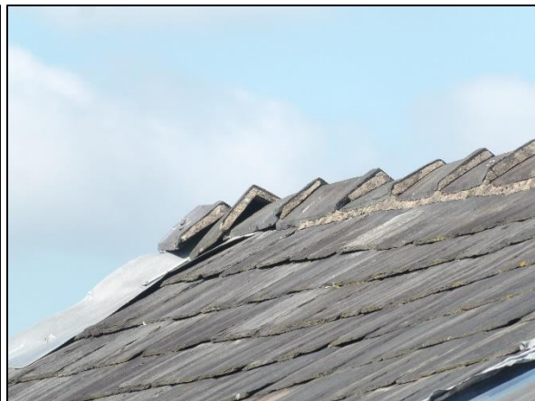
Figure 13: Dislodged ridge tiles and gaps under leadwork.
