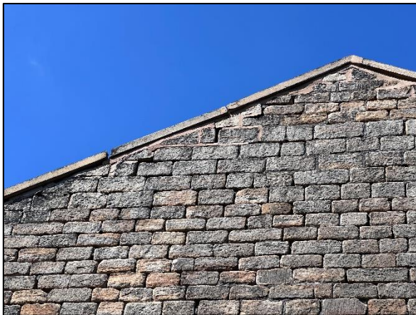
Figure 10: Voids in the stonework of the building.
