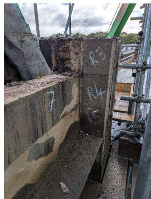
Displaced pilaster stone during dismantling.
