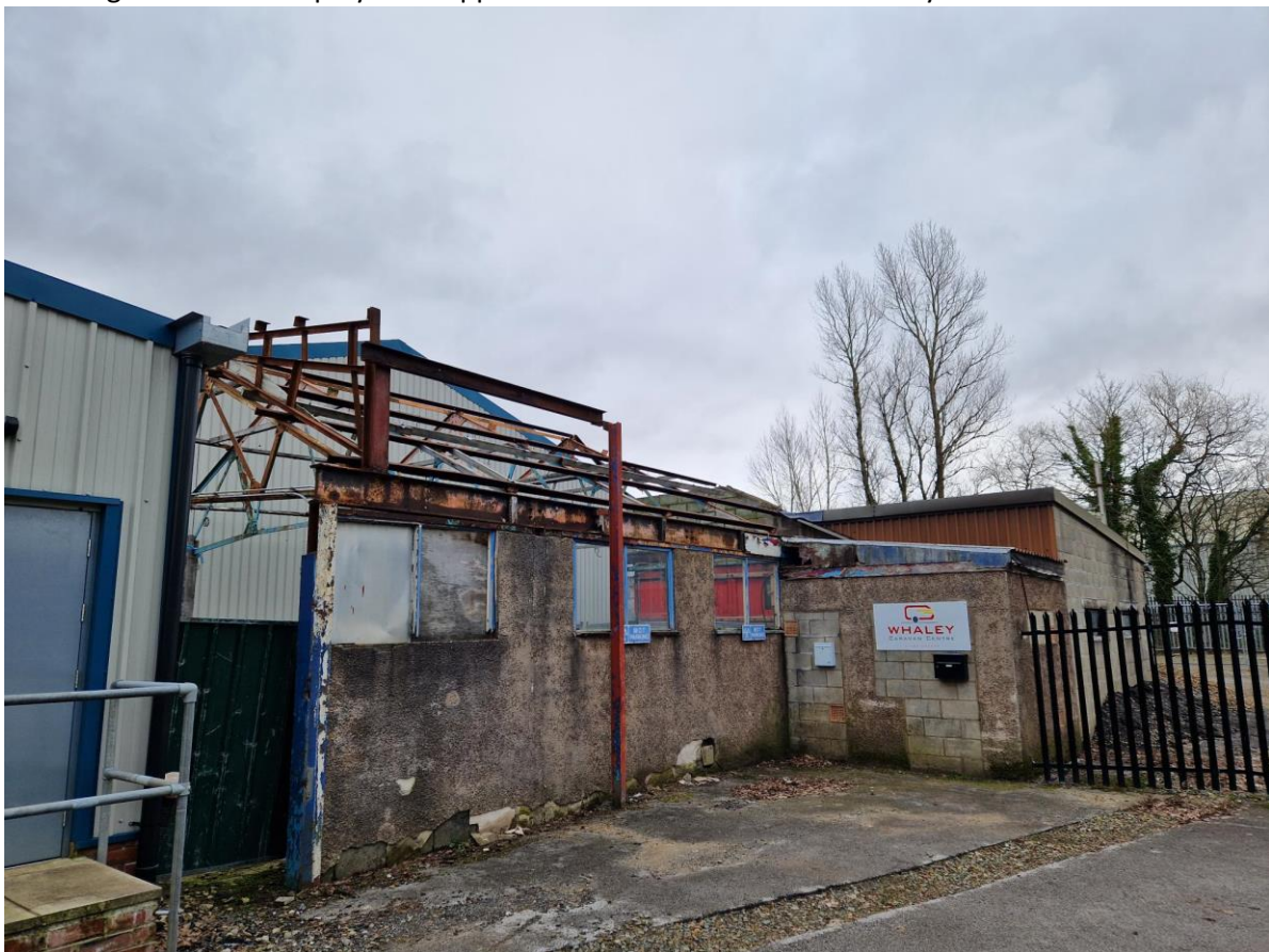
[Above – Photograph of the dilapidated structure adjoining existing units 2, 3 & 5]
