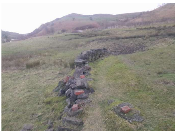
Photo 3: The partially collapsed drystone wall on the northern boundary of the site, viewed from the southwest.
