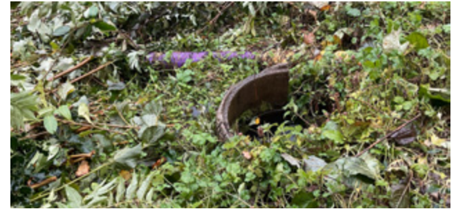
3.41a The Slopes, modern drainage pipe and tank
