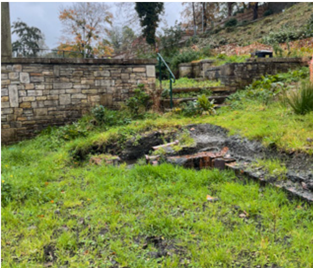
3.50 West garden area, exposed drains and brickwork
