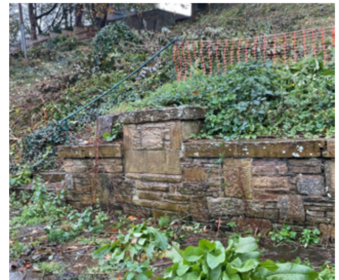
3.60 Possible lost plaque on the retaining wall to the gardens
