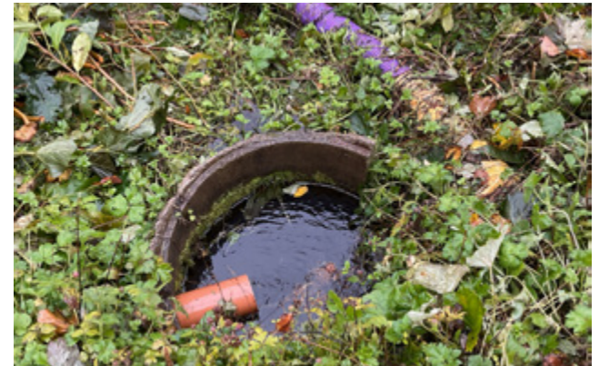
3.41b The Slopes, modern drainage pipe and tank
