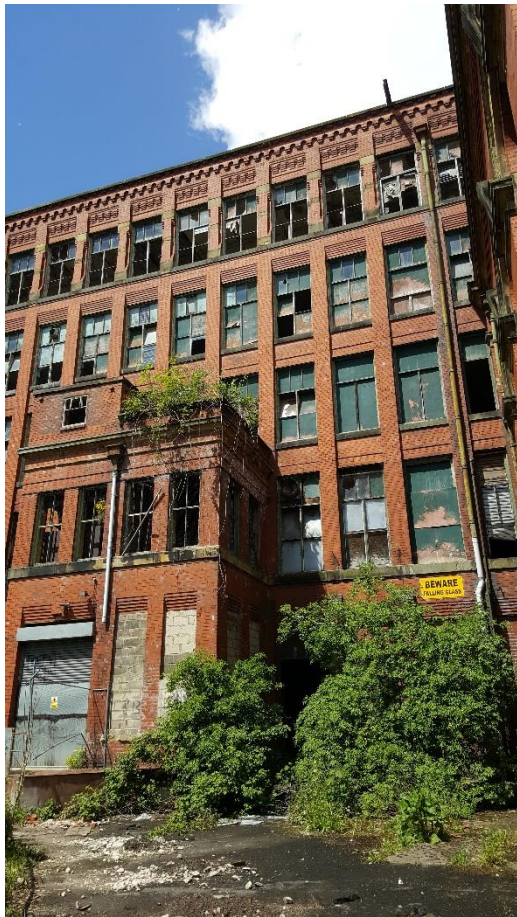
INFILLED WINDOW POSITIONS / WINDOW COMPONENTS LOST
