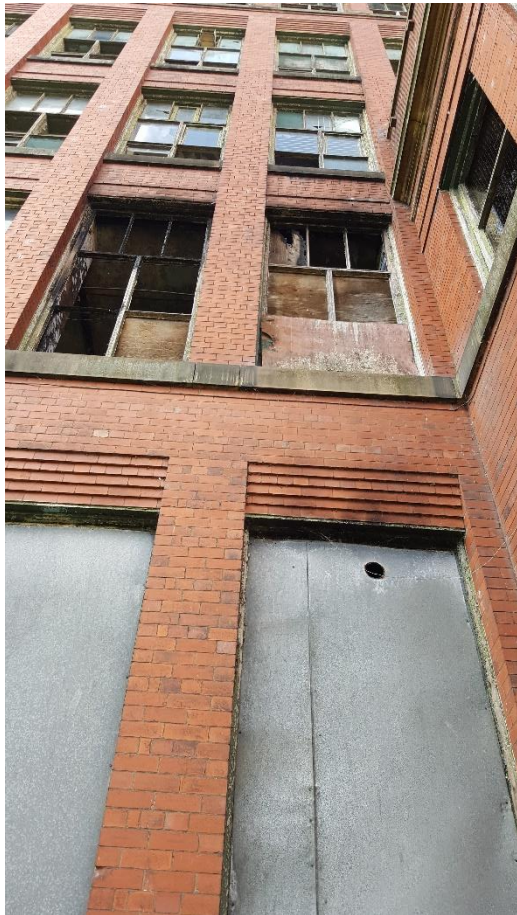
WINDOW COMPONENTS LOST/ GLAZING MISSING GIVING RISE TO TIMBER DECAY
