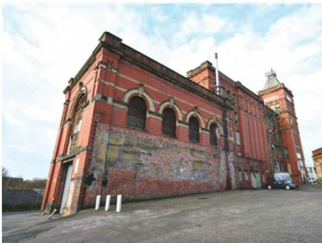
Engine house showing damaged facade
