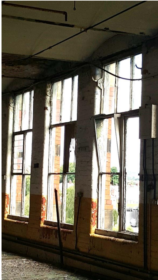
LOW CILL HEIGHTS/POOR VENTILATION HIGH LEVEL CONTROLS FOR RESIDENTIAL USE
