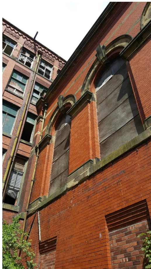
WINDOW DETERIORATION / MISSING INFILLED
