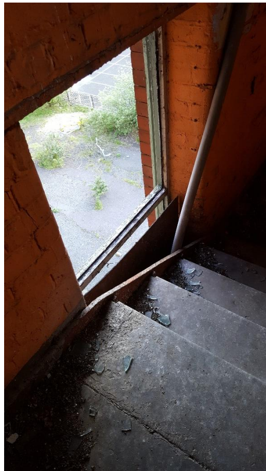
UNSAFE WINDOW ON MEANS OF ESCAPE ROUTE
