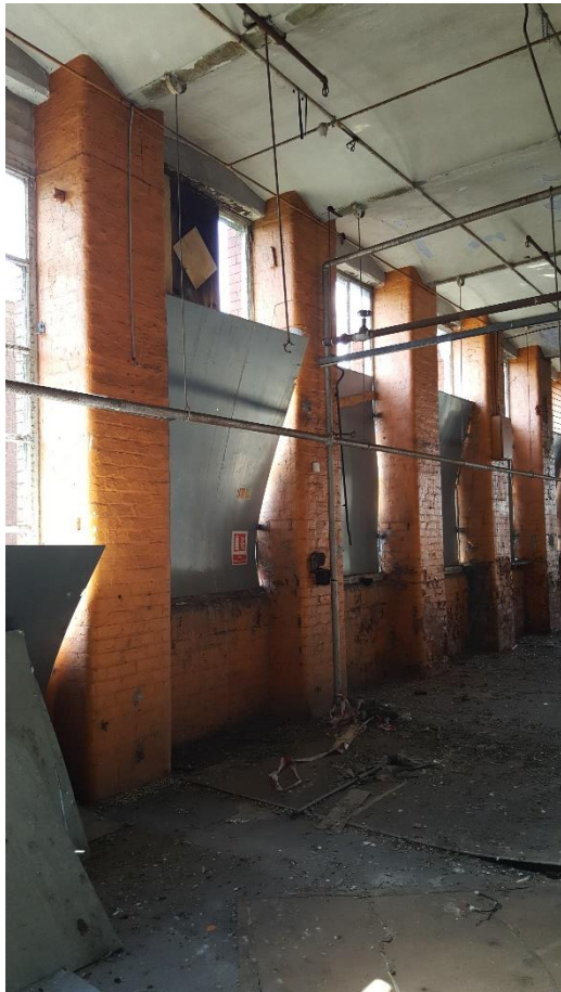
EXISTING WINDOW MISSING BEHIND PROTECTION
