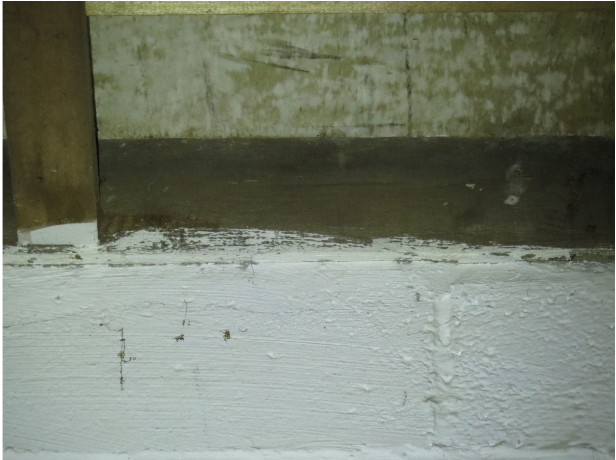
7 – There are no suitable gaps between roofing materials and blockwork.
