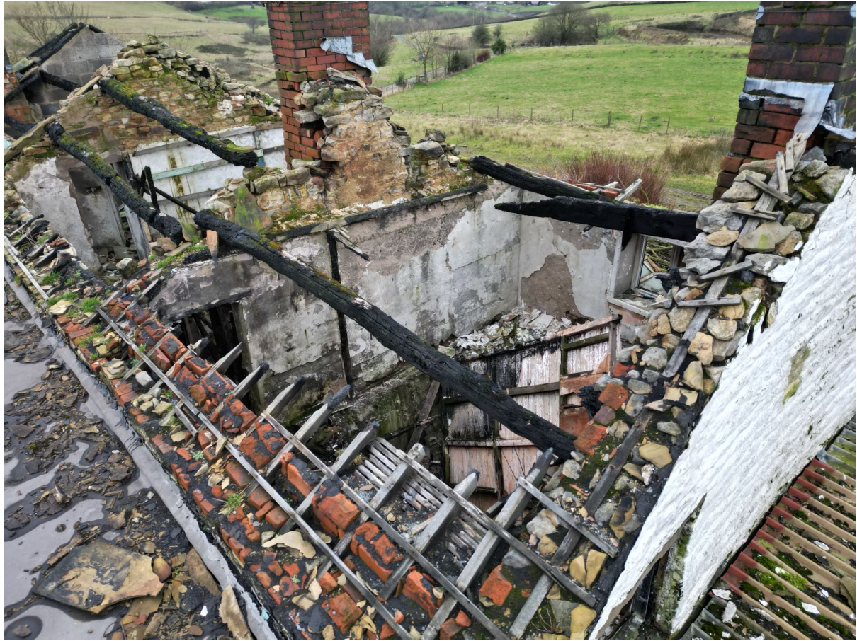
3 – The roof and inside of the building were destroyed by fire.
