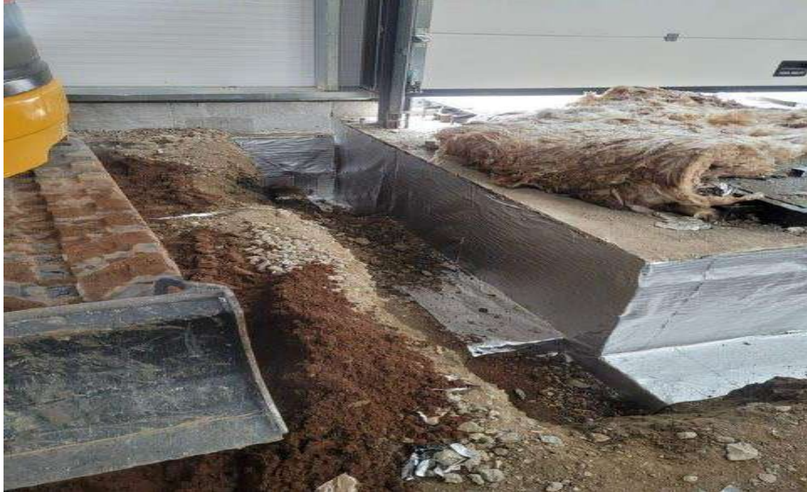
RTEC GRSAM (Silver) Unit M2 docking bays
